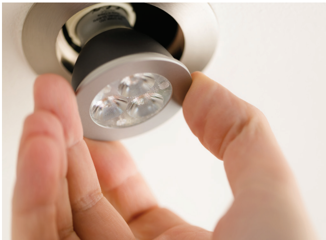
LED light bulb installed into a ceiling can fixture.
