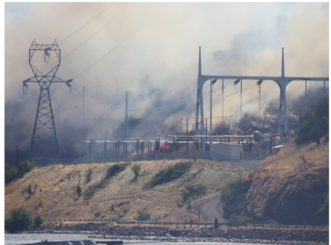
A wildfire burns near a BPA right-of-way and substation.
