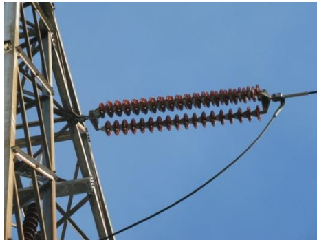
230 kV Line Dead End
