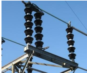
230 kV Disconnect Support
