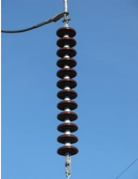
230 kV Riser Bus in Bridge
