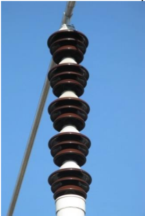
230 kV Bus Support
