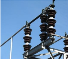
115 kV Disconnect Support
