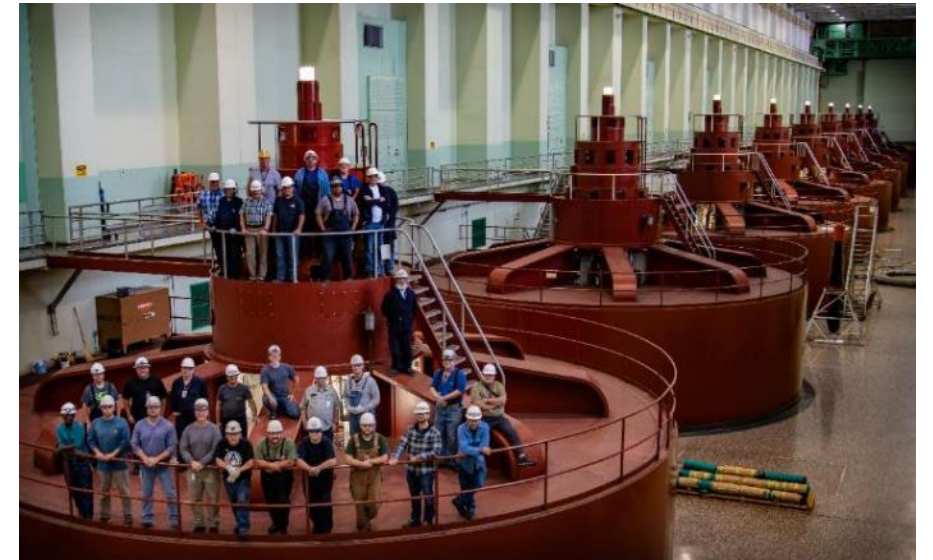
FY18 Grand Coulee Right Power House (9 units online)
