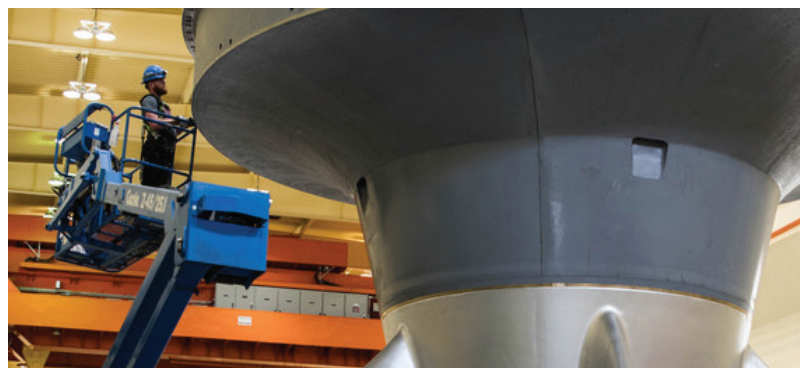
New high-tech turbines at Ice Harbor Dam improve safety for fish, and produce more power.
