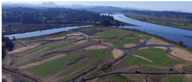
Removing old agricultural dikes at the confluence of the Wallooskee and Youngs rivers near Astoria, Oregon, to allow water to inundate the historic floodplains and improve habitat for young fish on their way to the ocean.
