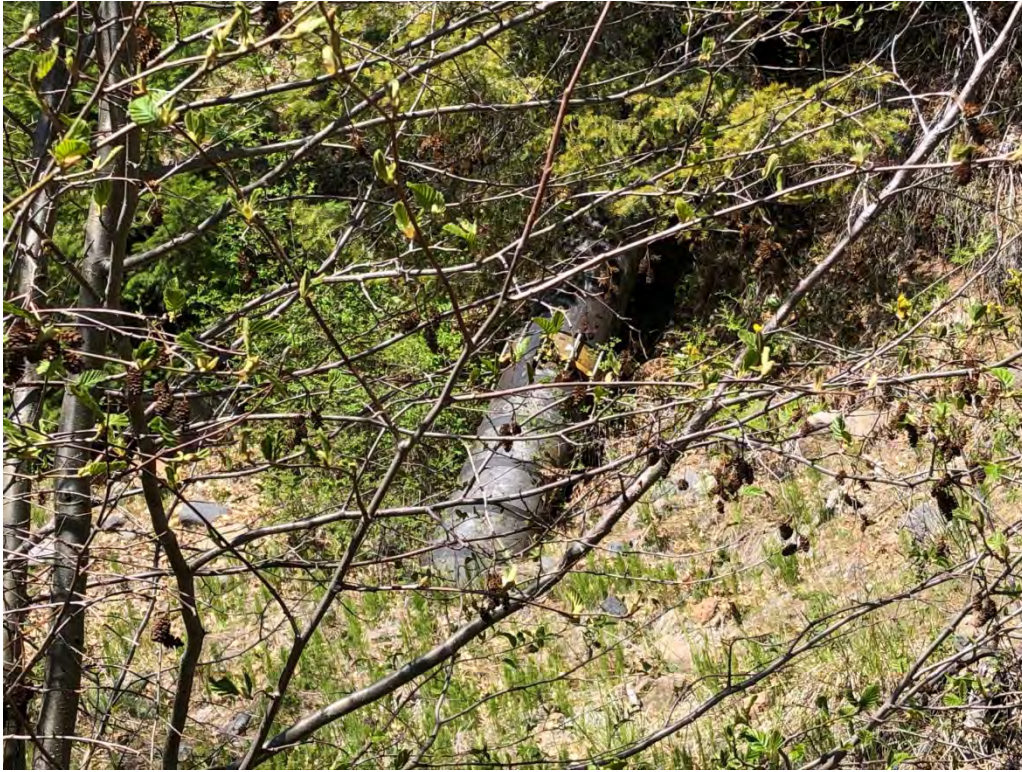
Photo 11. Looking north at lower intake pipe that lies adjacent to Indian Ford A Spring.
