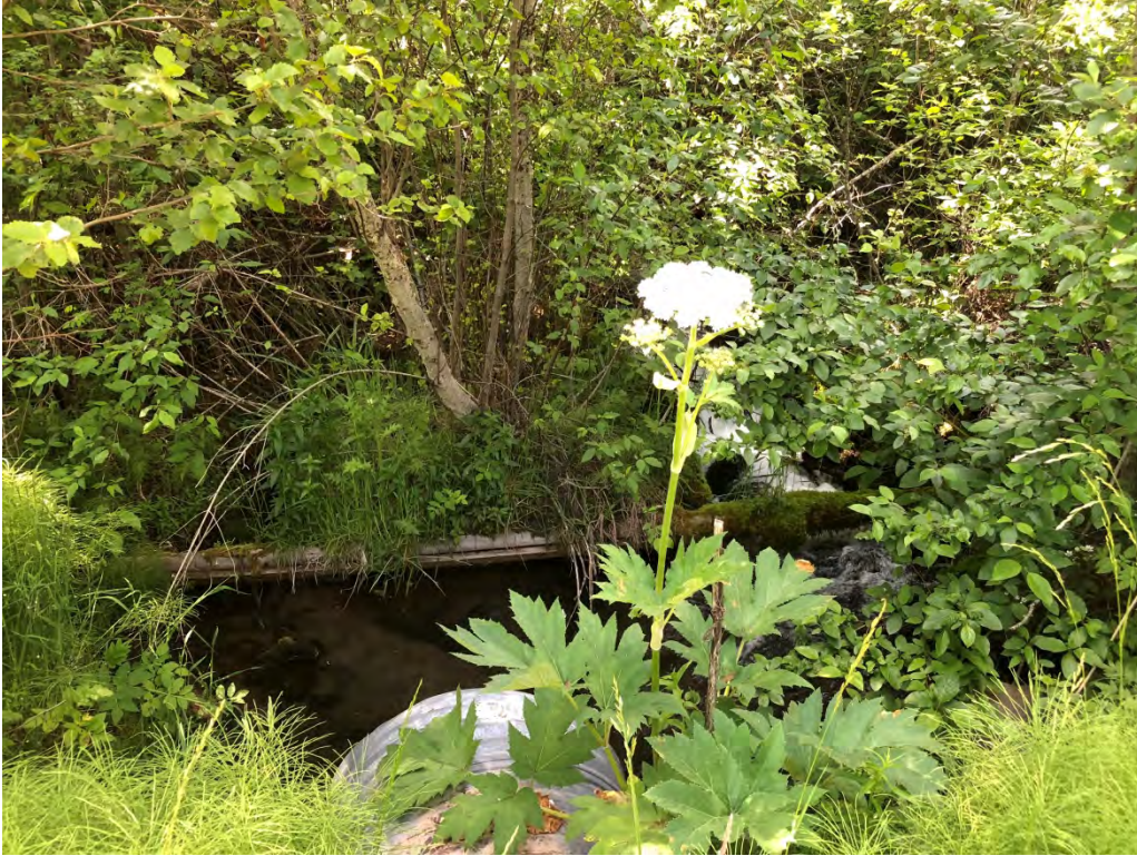
Photo 9. View of culvert near at the base of Indian Ford A Spring that flows into the Klickitat River.
