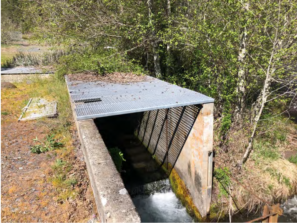
Photo 17. View of outlet to fish ladder where it flows into the Klickitat River.
