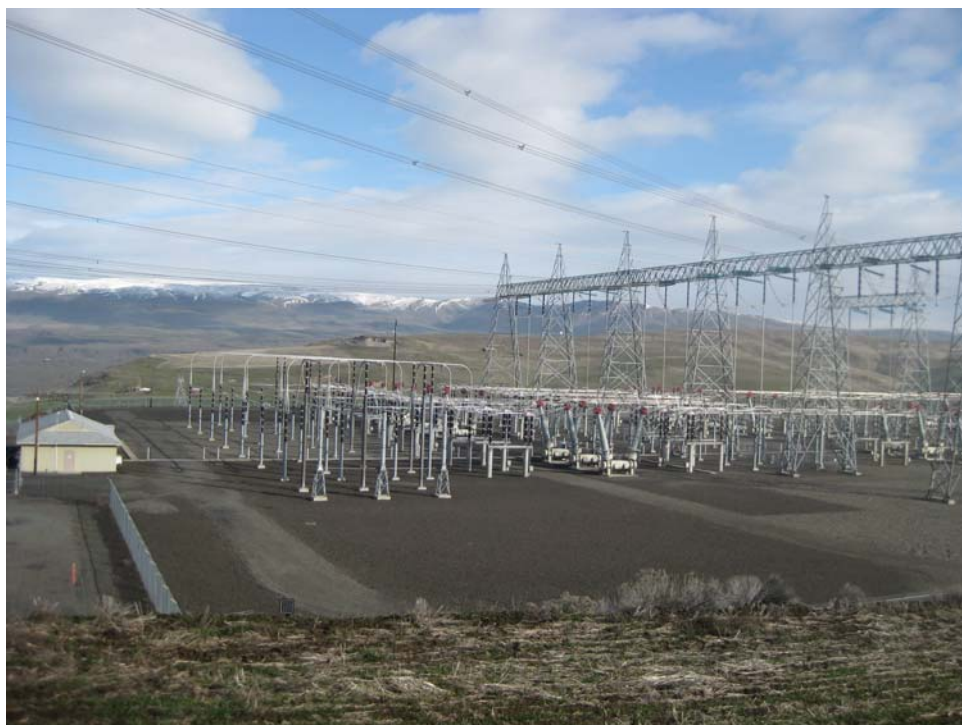
Typical 500-kV Substation
