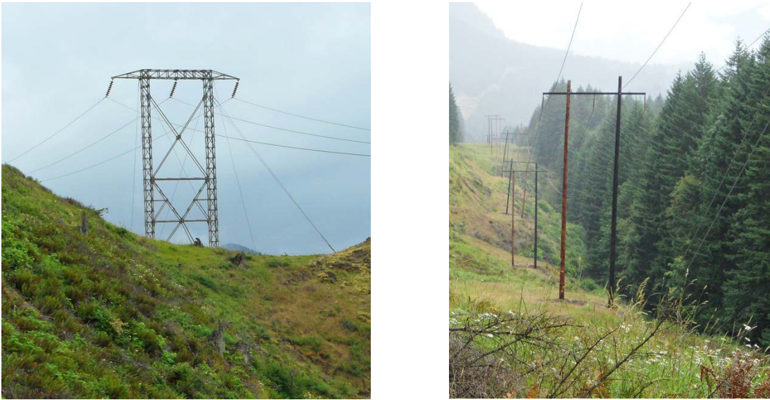
Figure 2.1-2. Photos of Existing Lattice-steel H-frame and Wood-Pole H-frame Structures along the Bonneville-Hood River Line
