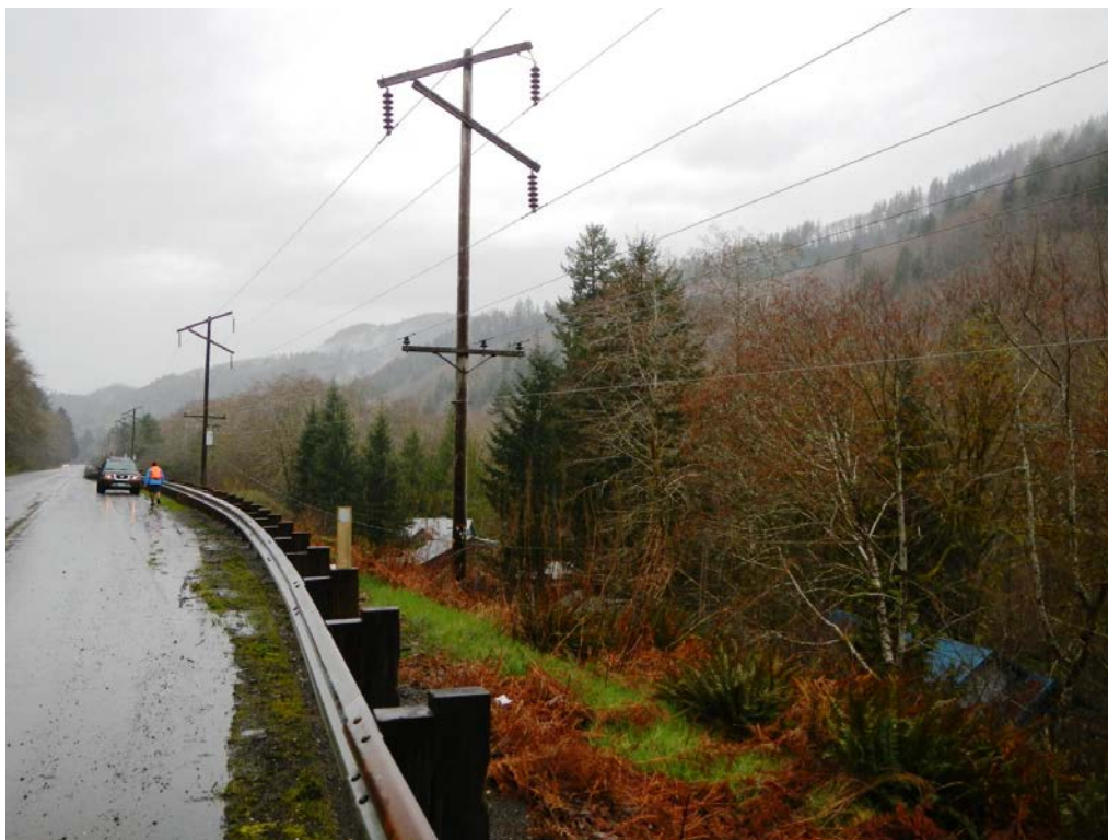
Figure 2-1. Existing Forest Grove-Tillamook No. 1 Transmission Line
