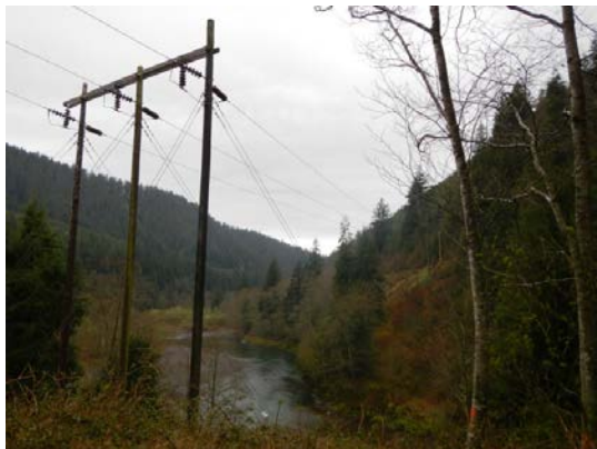
At structure 54/2 (Forest Grove-Tillamook No. 1). Transmission line crosses over the Wilson River. Blackberry thicket under lines. Danger trees on right, small alder trees marked with orange paint.
