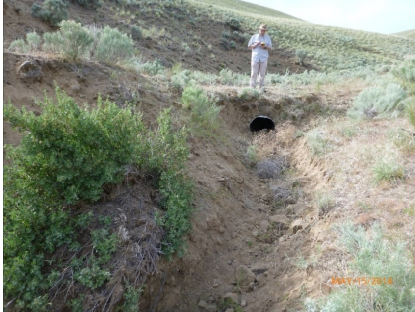
Figure 3.10-4. Photograph shows an existing culvert in an ephemeral stream between Midway-Grandview Structures 12/3 and 12/4 in Line Mile 12 that would be replaced. (Source: Tetra Tech 2014d)
