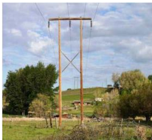
Figure 2-11. Danger Trees Near Midway-Moxee Structure 30/3
