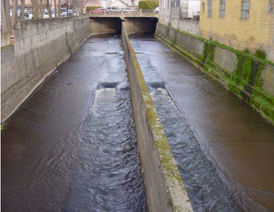
Figure 8. Reach Type 7, Rectangular Split Flume (Photo provided by Tri-State Steelheaders)
