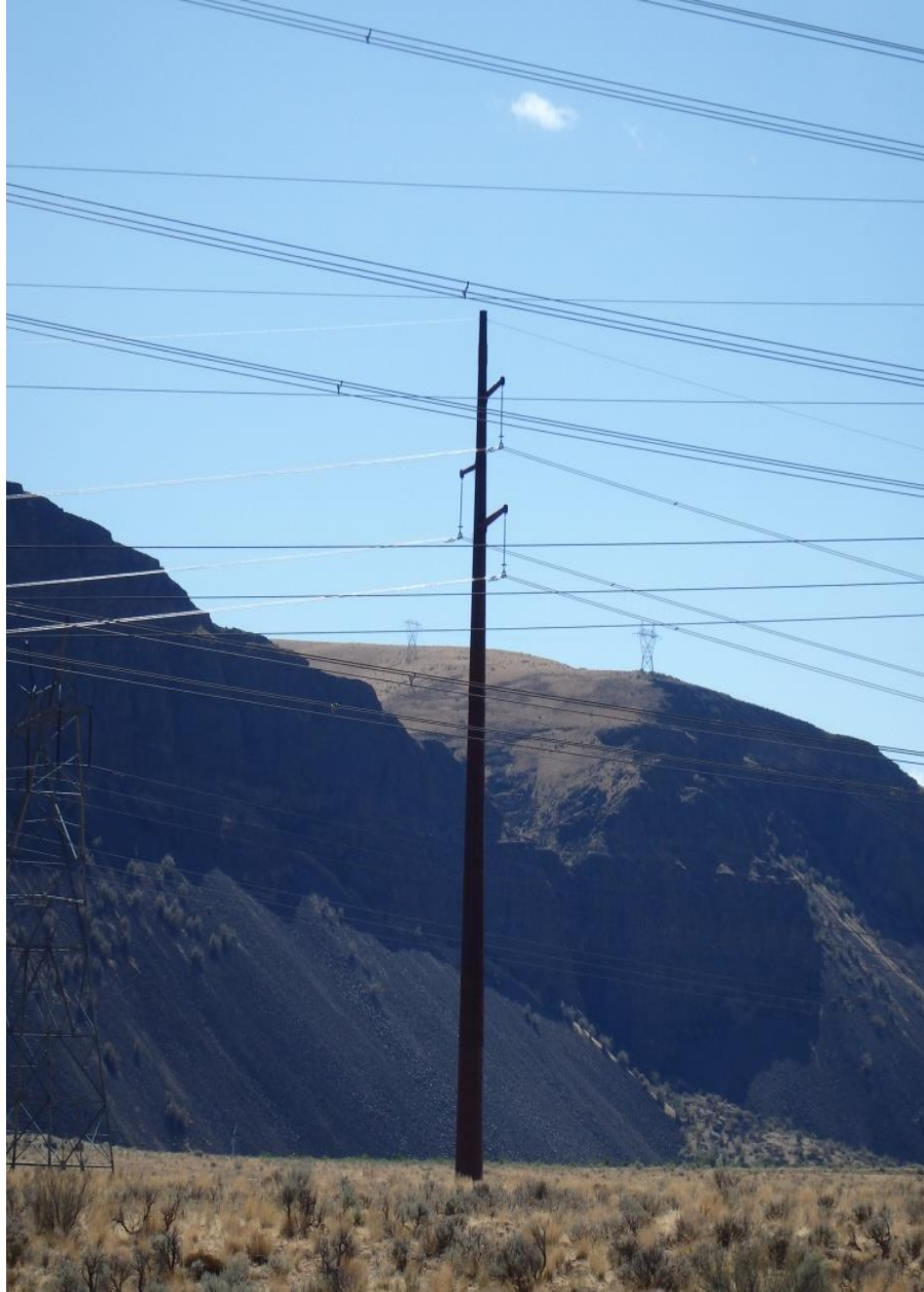
Photo 3.10-10. Recently constructed Douglas PUD transmission line with the same type of steel-pole structures that would be used for the proposed Rapids-Columbia transmission line
