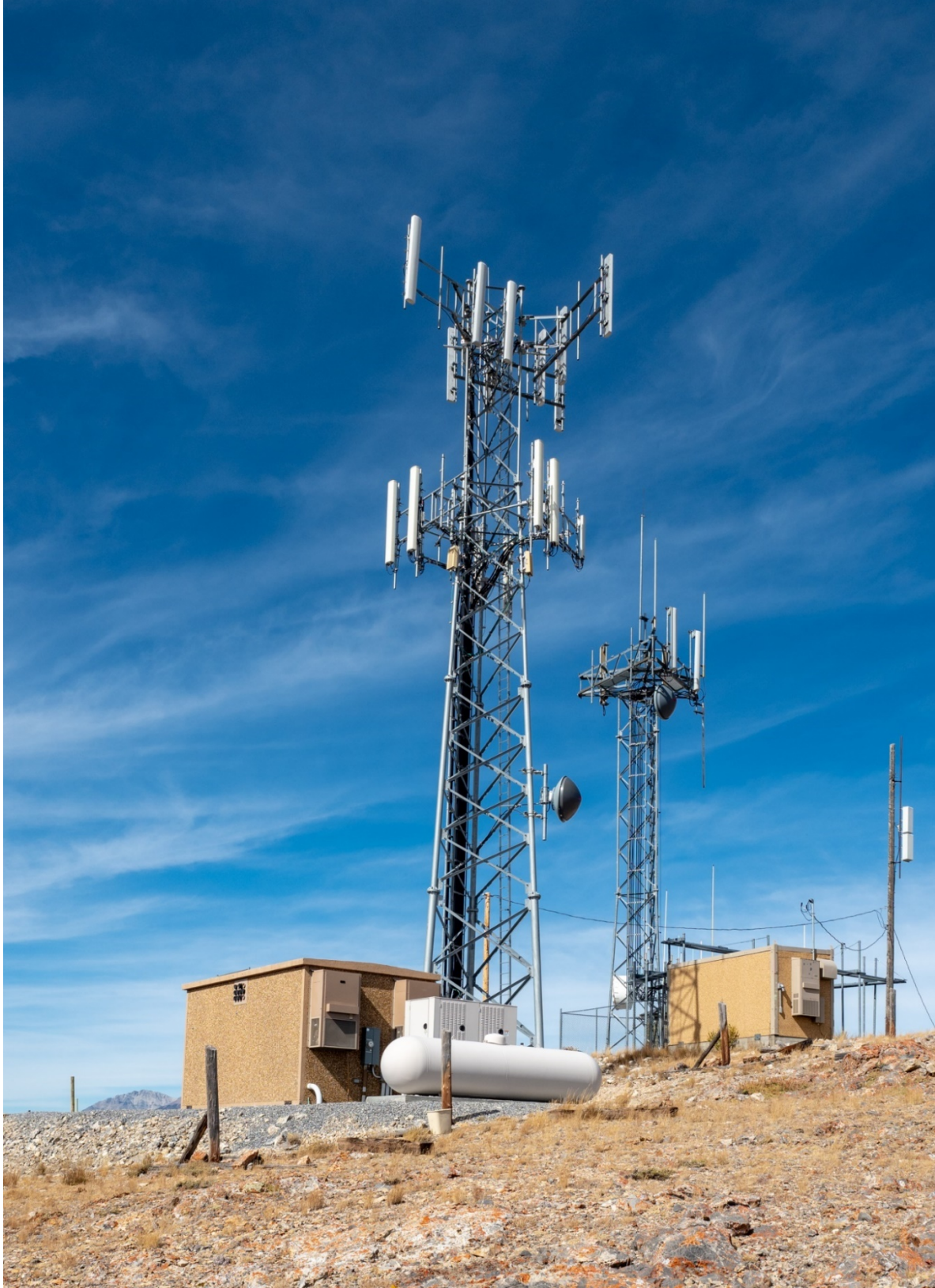
Figure C1-5. Windy Devil Existing Communication Station
