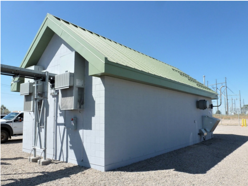
Figure C1-2. Example of a Typical BPA Communication Station
