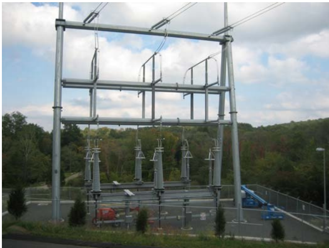
FIGURE 2-13 TRANSITION STATION AND STRUCTURES (WPSC PHOTO)
