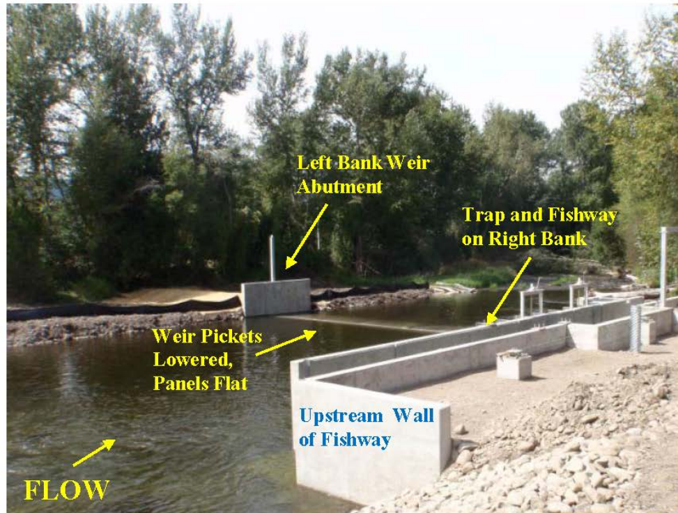
Figure 5. Photographs of the Lostine River Satellite Facility Weir and Fishway/Trap in Lostine, Oregon (immediately post-construction, plantings not yet established along banks).
