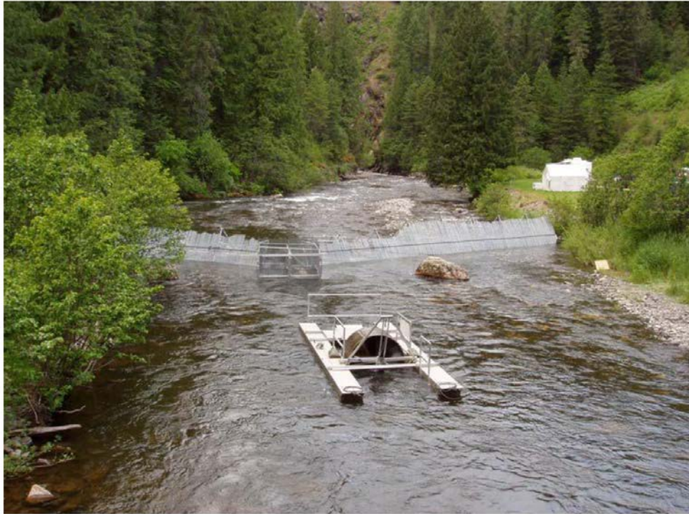
Photo 1. Nez Perce Tribe Lower Lolo Creek trapping site located on BLM property. Rotary screw trap in front, temporary picket weir in back, workup tent and camp trailer on north (right) bank. Proposed weir would be located slightly upstream of the picket weir location shown in this photo.
