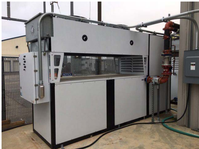
2 Glycol Chillers - 40 Tons Total
