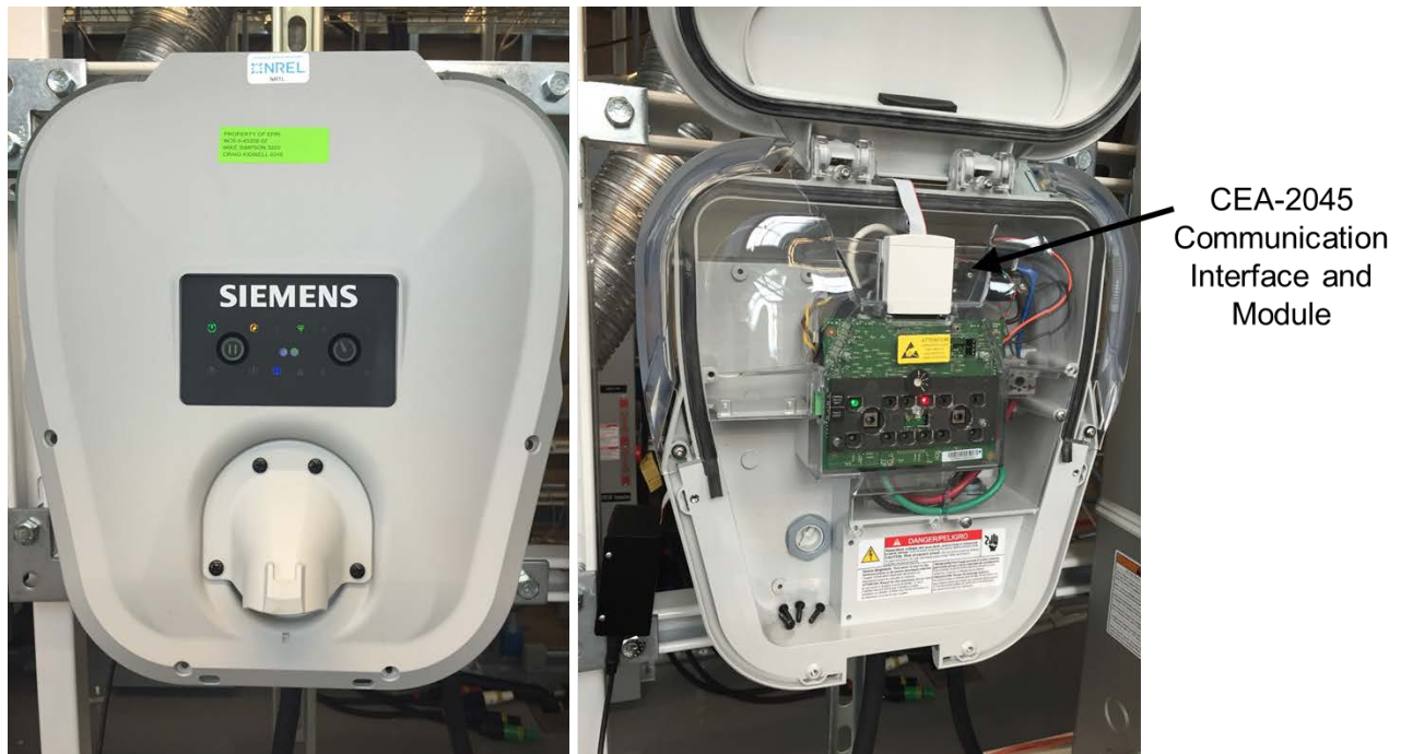
Figure 2-2 EVSE Installed at NREL
