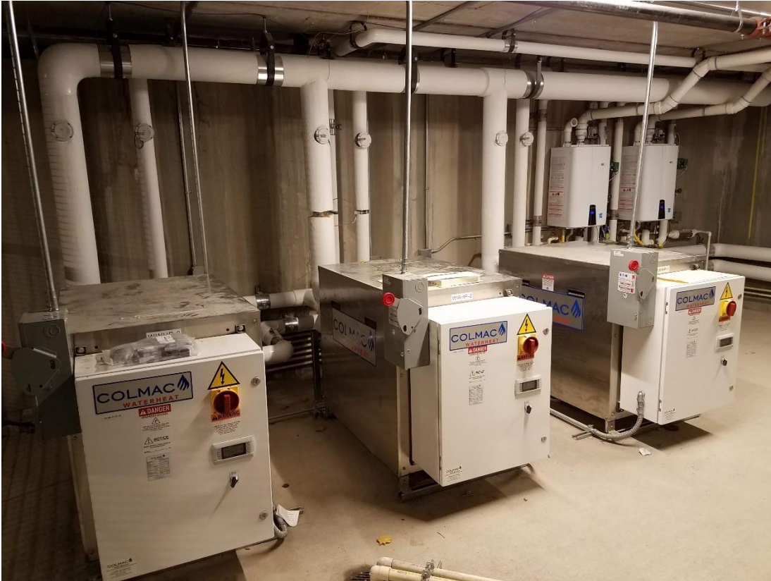
Figure 6. Water-to-Water Heat Pumps: Colmac HPW12 primary heaters with gas water heater back-up equipment mounted on the wall
