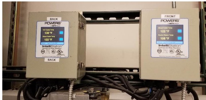
Figure 10. Read-out from digital missing station (TMV-1) during system commissioning
