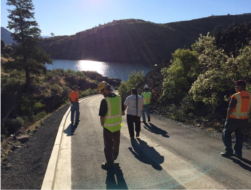
Figure Q-7. The final inspection at the completed Eden Harbor Pictograph stabilization.
