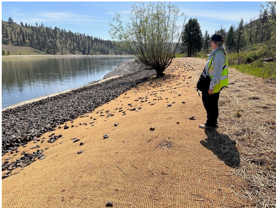
Figure K-7. Site 45LI377 Stabilization Project showing large gravels placed above the cellular system, covered with topsoil and native plantings in areas above the ordinary high-water mark.
