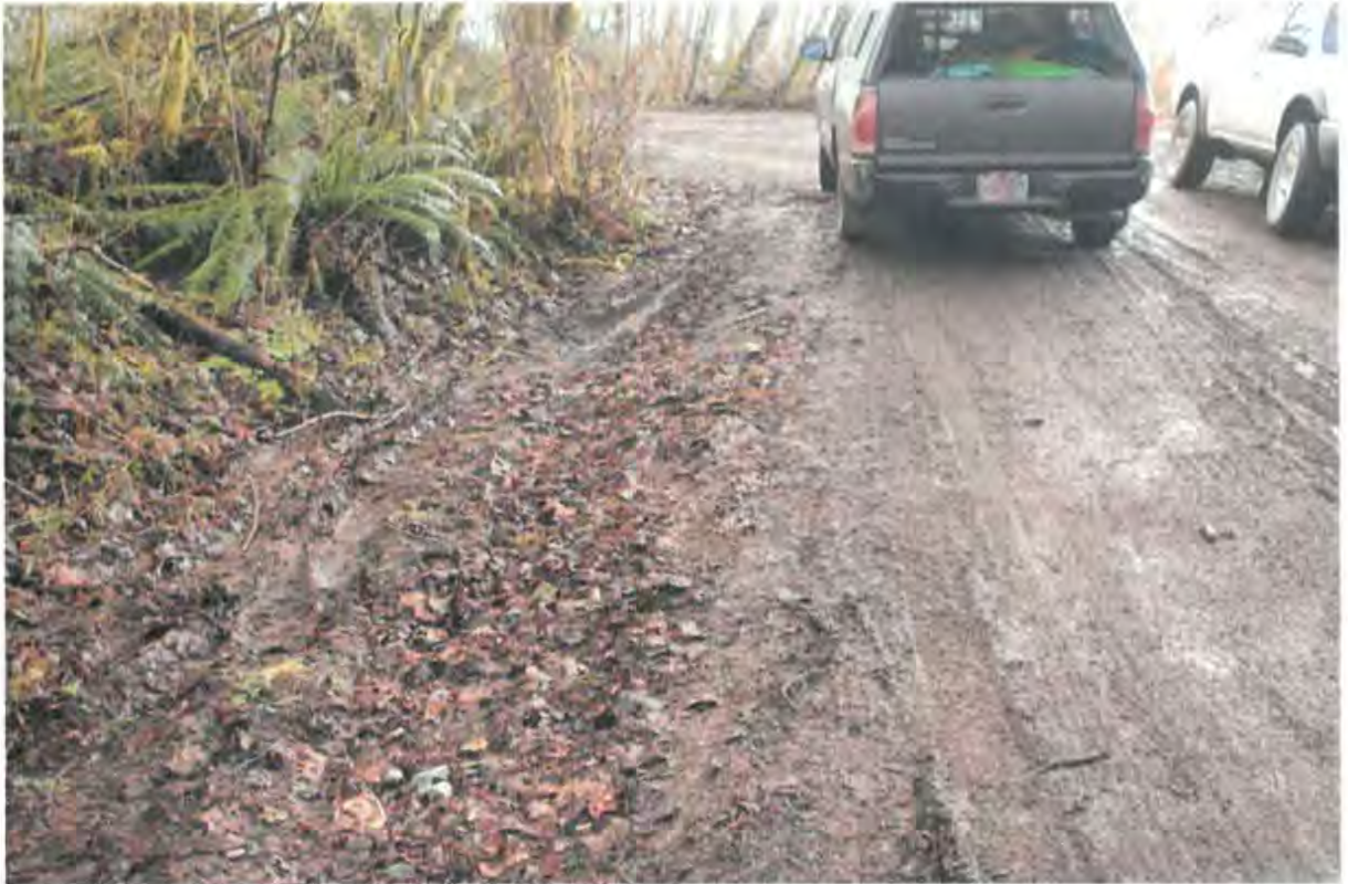
Roadway conditions with a thick layer of accumulating debris evidenced by the depth and mushiness of the tire tracks in the roadway
