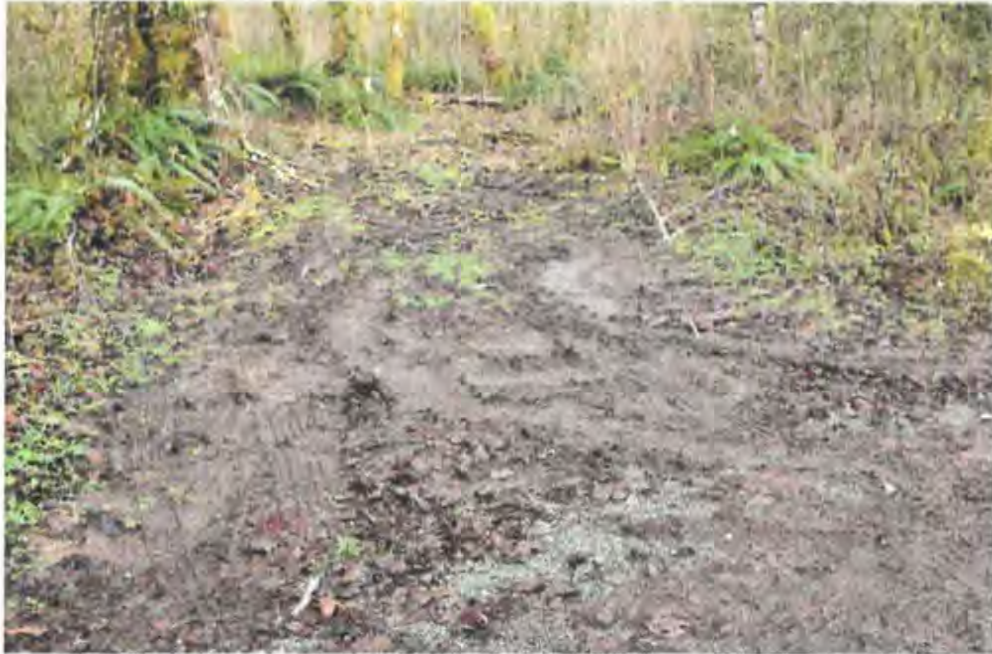
Designated parking is un-graveled. The patchy gravel is the roadway covered with accumulating debris
