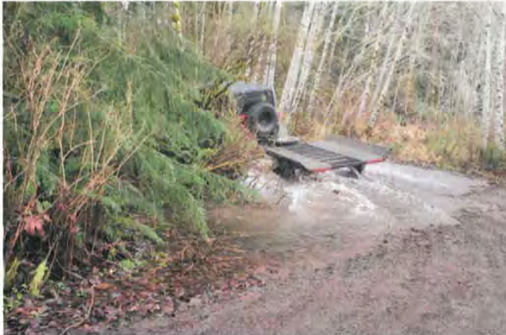
Drainage problem and water flowing over the roadway
