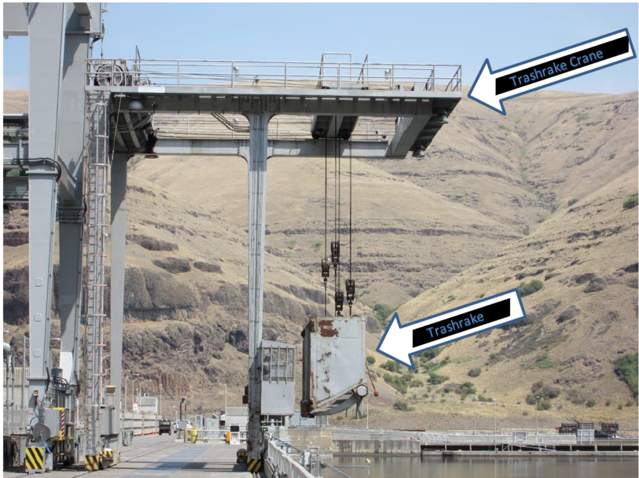
Lower Granite dam and reservoir project's Trashrake Crane and Trashrake
