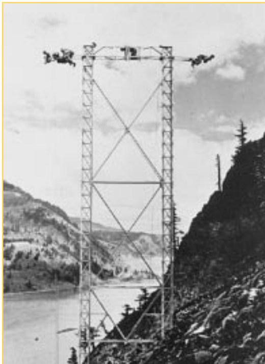
Building the tower along Shell Rock Mountain for the Bonneville-The Dalles Line, 1941.
