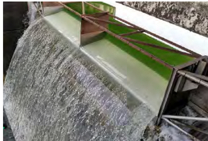
Foster Spill Weir for downstream fish passage - 2018
