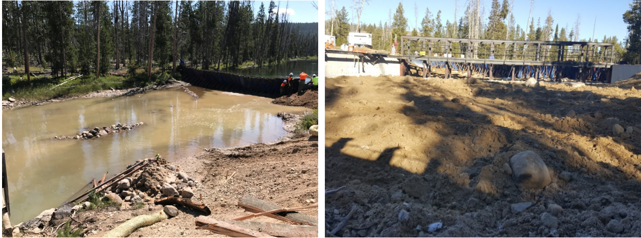
Figure 17 Example of short-term direct effects of instream work during Redfish Lake Creek weir construction
