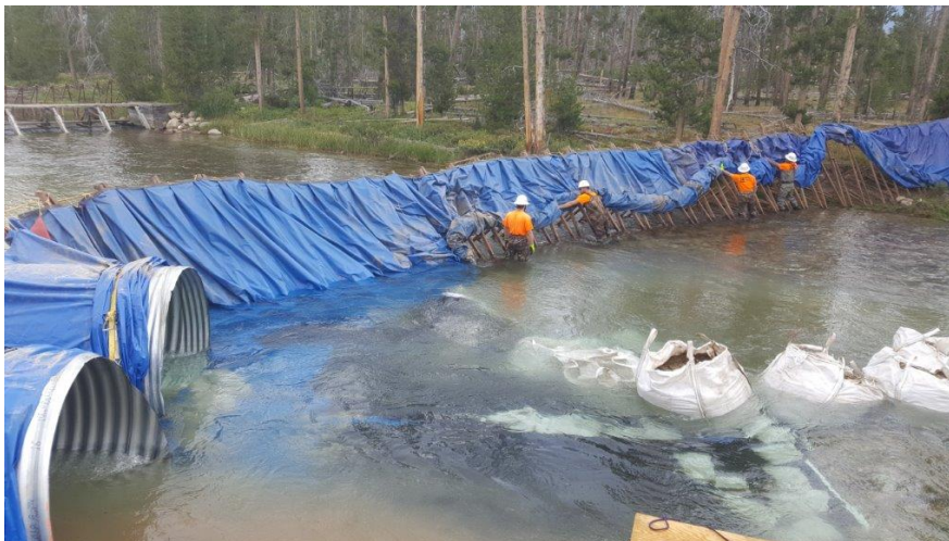
Figure 15 Example of coffer dam and bypass pipes for Redfish Lake Creek weir construction
