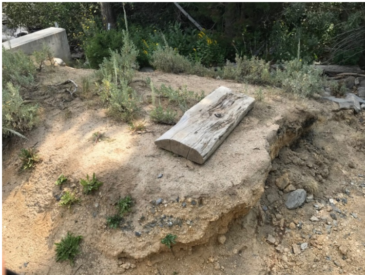
Figure 6 Washout in area at end of proposed access road to right bank abutment (current abutment visible in upper left)
