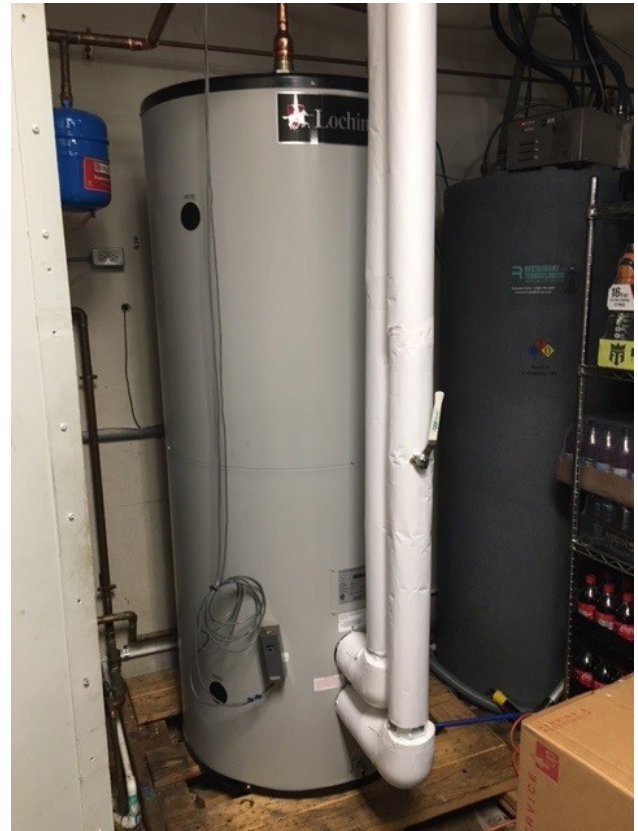
Figure 5. Multipass piping into tank.
