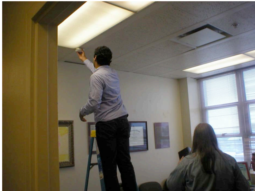
Figure 5. Installation of the Wattstopper IT-200 IntelliTimer® Pro Logger
