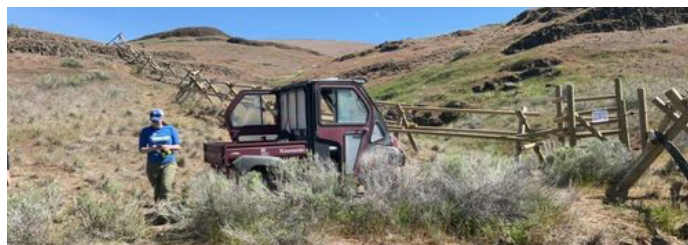
Installation of a buck-and-rail fence and gate to discourage recreational impacts to a site at Lower Granite in FY 2022.
