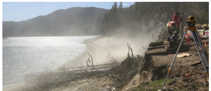
Excavation of an eroding bank at 45ST1111 on the Mainstem of Lake Roosevelt in FY 2022.
