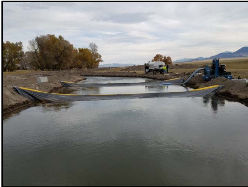
2017084 (Pahsimeroi Page): A 90 foot long 8 foot deep settling pond at the downstream end of the bypass channel. Two sediment curtains were also installed in order to reduce fines in the river.
