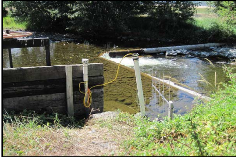
2017013: Tully Hill Channel Spanning Barriers (Before)
