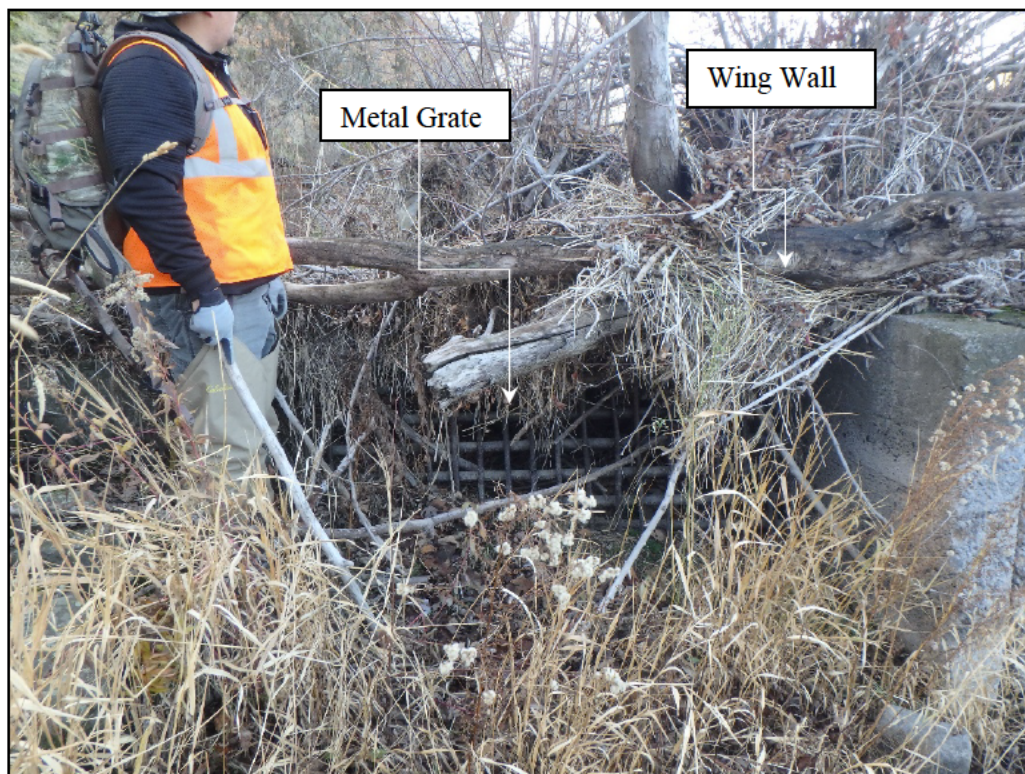
Photograph 5. Close-up looking west of the grate in the headgate and the concrete wing wall in the right frame (18-128:4). 12/12/2018.
