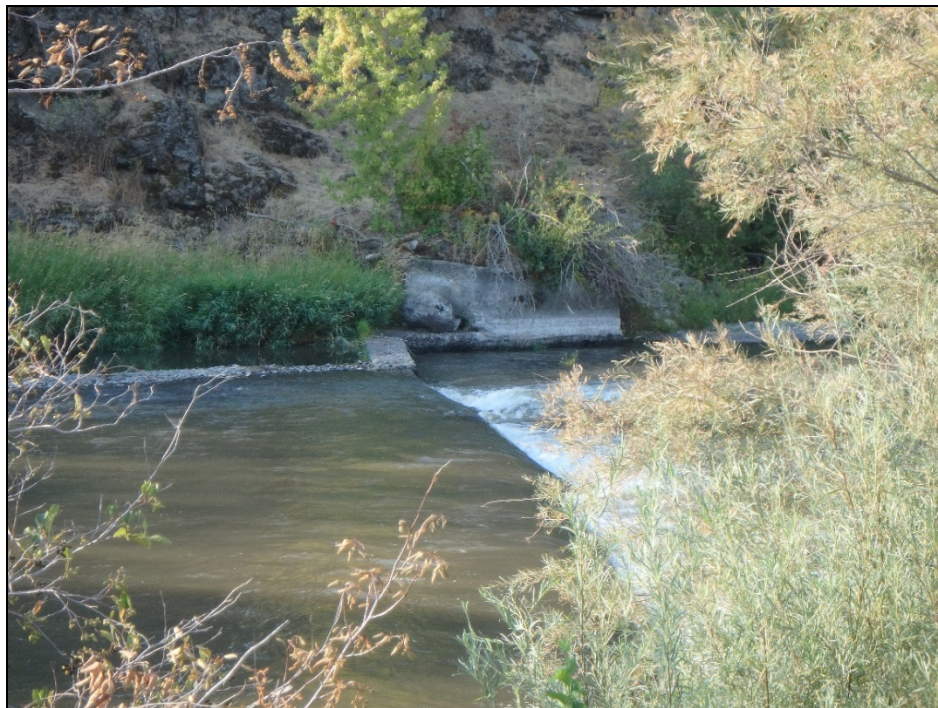
Photograph 4. View at 157° of the south side of the dam showing concrete wing wall and the location of the former diversion (full of green vegetation; 18-106:29). 9/7/2018.
