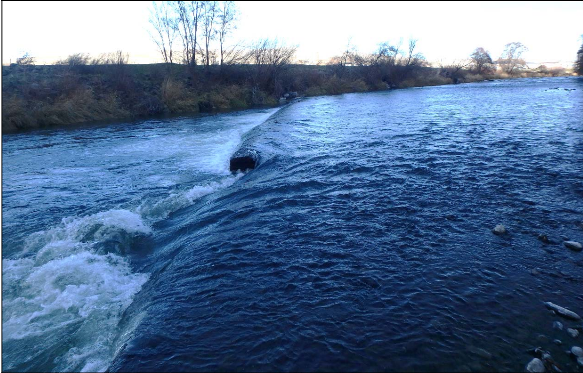
Photograph 3. View at 341° of the dam from the south side of the Umatilla River (18-128:1). 12/12/2018.
