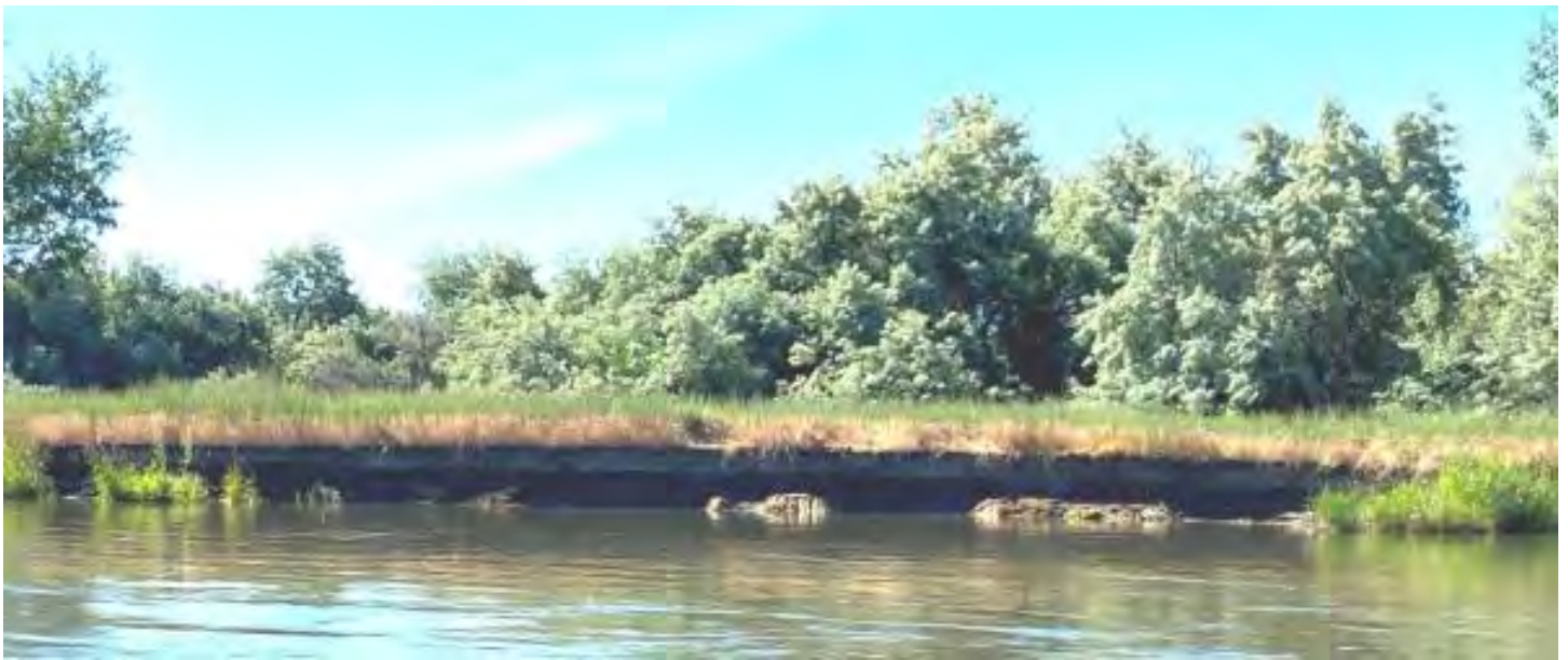
Erosion along bank
