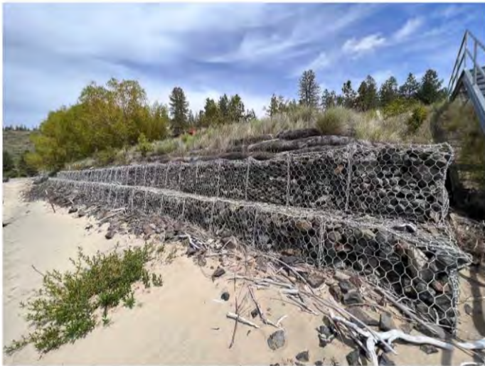
Figure 7. 45-ST-11 shoreline stabilization system.
