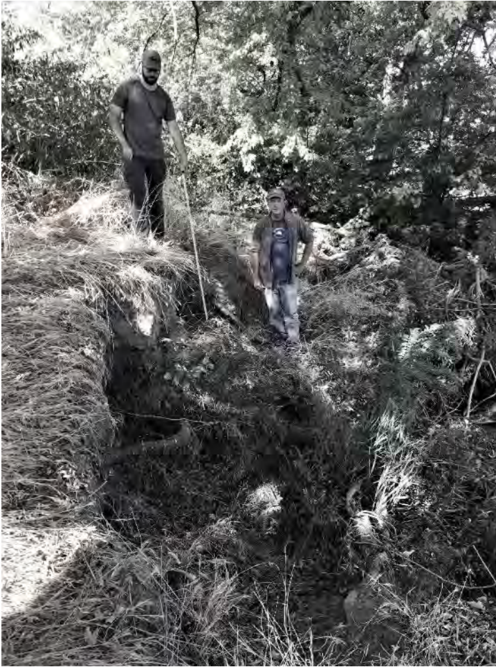
Figure F-1. Corps visit at McNary site 45WW13 in FY 2021 to measure the amount of clean fill material needed to fill an area of excavated/eroded bank.
