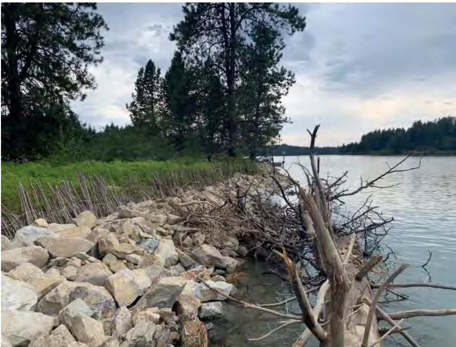
Figure H-5. Live willow stakes were placed between the natural bank and riprap. Willows will help to shade the shoreline and protect fish habitat.
