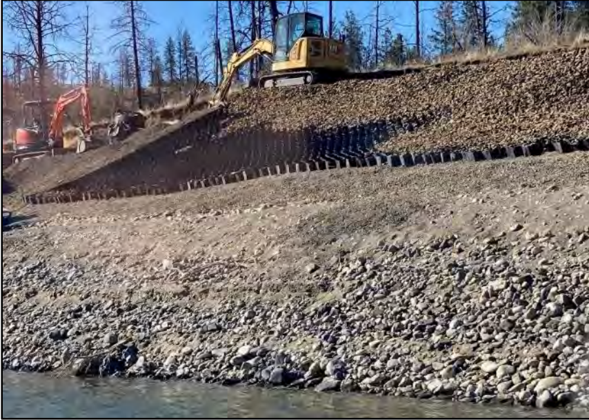
Figure J-5. Stabilization of 45LI377 in progress during spring 2021. The cellular containment system is being filled with crushed rock and overlaid with topsoil for later planting.
