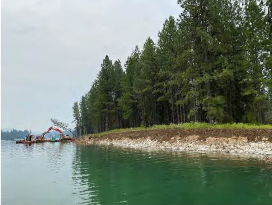
Figure H-6. Bank stabilization is nearly complete with contractor placing the final layer of mulch to help ensure the longevity of willows and other species of native riparian vegetation.
