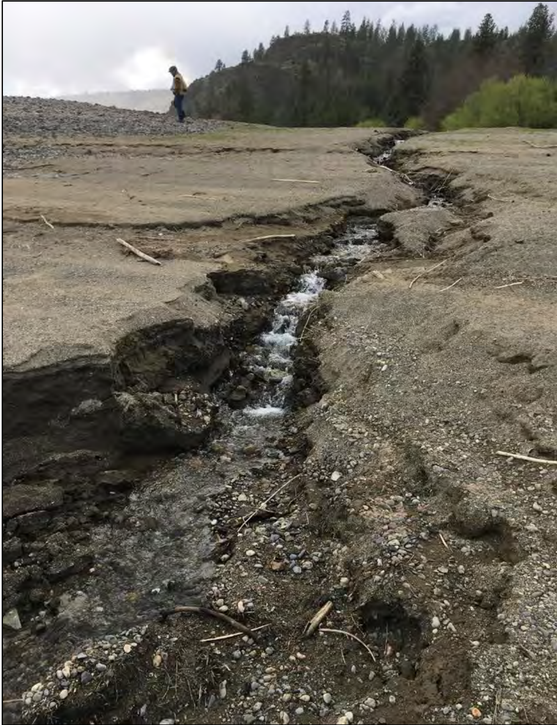
Figure J-9. STIPP staff assessing erosion at a site on the Spokane Arm during the Spring 2021 Site Condition Monitoring fieldwork.
