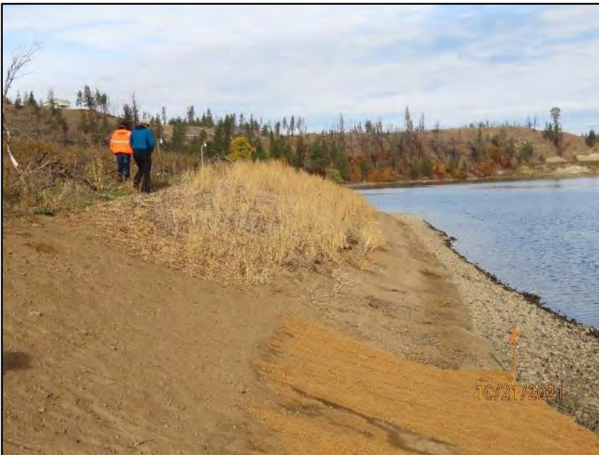
Figure J-6. Reclamation staff inspect upstream end of Phase 1 at 45LI377 after completion.
