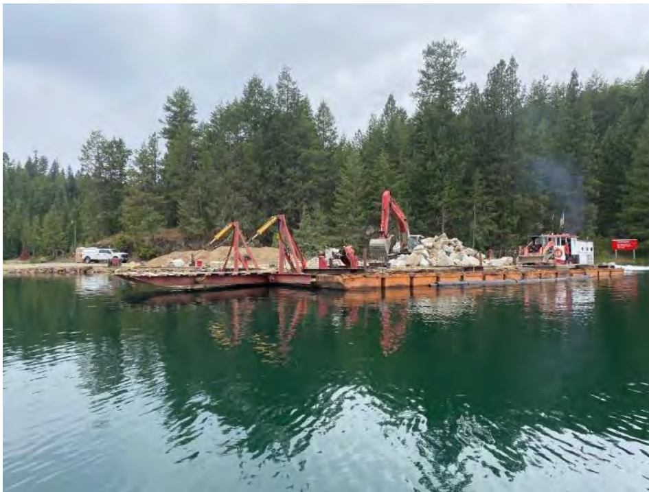
Figure H-3. Materials for bank stabilization were staged at nearby recreation area.
