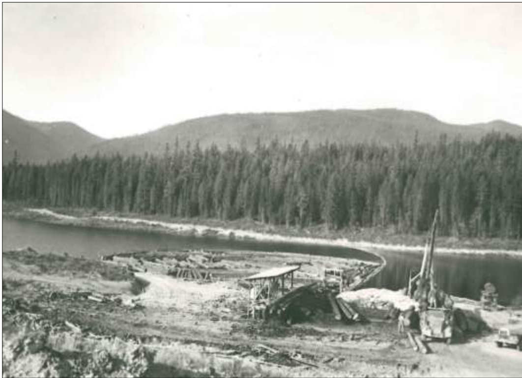
Figure 25 Removing logs from the reservoir at Emery Creek. Source: BOR Project History, 1956, National Archives, Denver.
