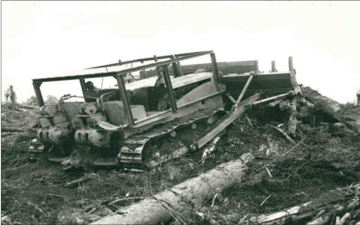
Figure 18 “Twin D8’s” clearing timber on the Hungry Horse Project. Source: BOR Project History, 1950, National Archives, Denver.
