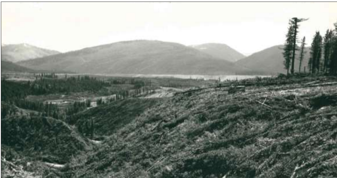
Figure 11 Caterpillar tractor clearing steep terrain. Source: BOR Project History, 1950, National Archives, Denver.
