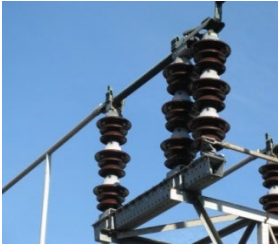
115 kV Disconnect Support
