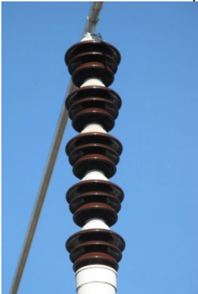
230 kV Bus Support
