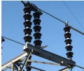
230 kV Disconnect Support
