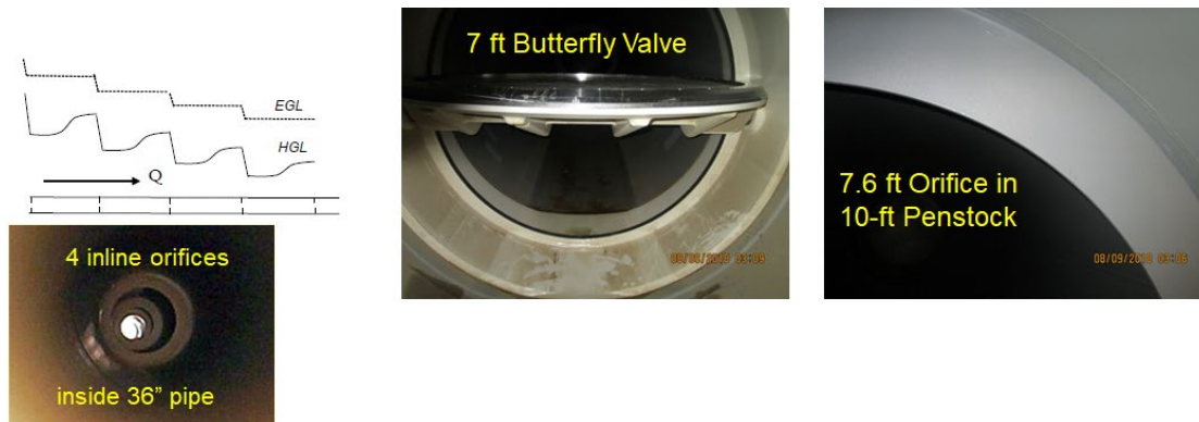
Figure 2-14. In-line Orifice Systems inside Pipelines (Seven Oaks Dam, lower left; The Dalles Dam, upper middle and right)
