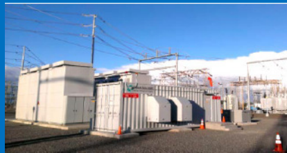
Vaca-Dixon BESS 2 MW / 14 MWh NAS Battery Vaca-Dixon Substation
