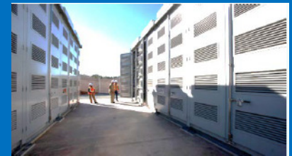
Yerba Buena BESS 4 MW / 28 MWh NAS Battery Customer R&D Facility, San Jose
