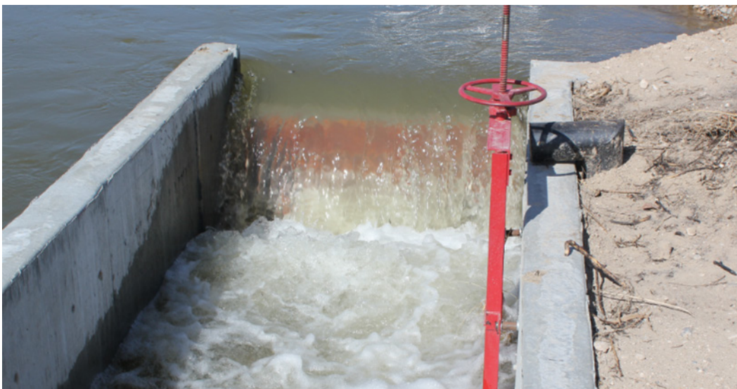
South Columbia Basin Irrigator District automated canal gates.
