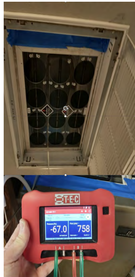
Figure 5. Total Air Handler floor test.
