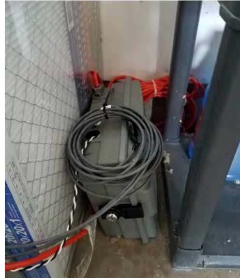
Figure 14. Elite Logger (inside gray box) next to indoor fan.
