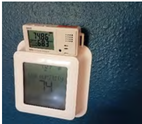
Figure 8. Central Thermostat and Temperature Logger
