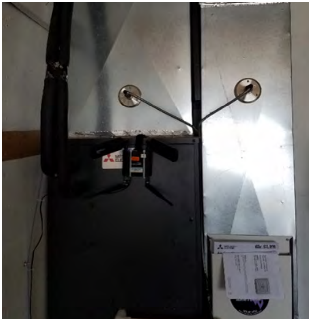
Figure 13. Internet Cell Modem (AT&T) and temperature probes in supply ducts
