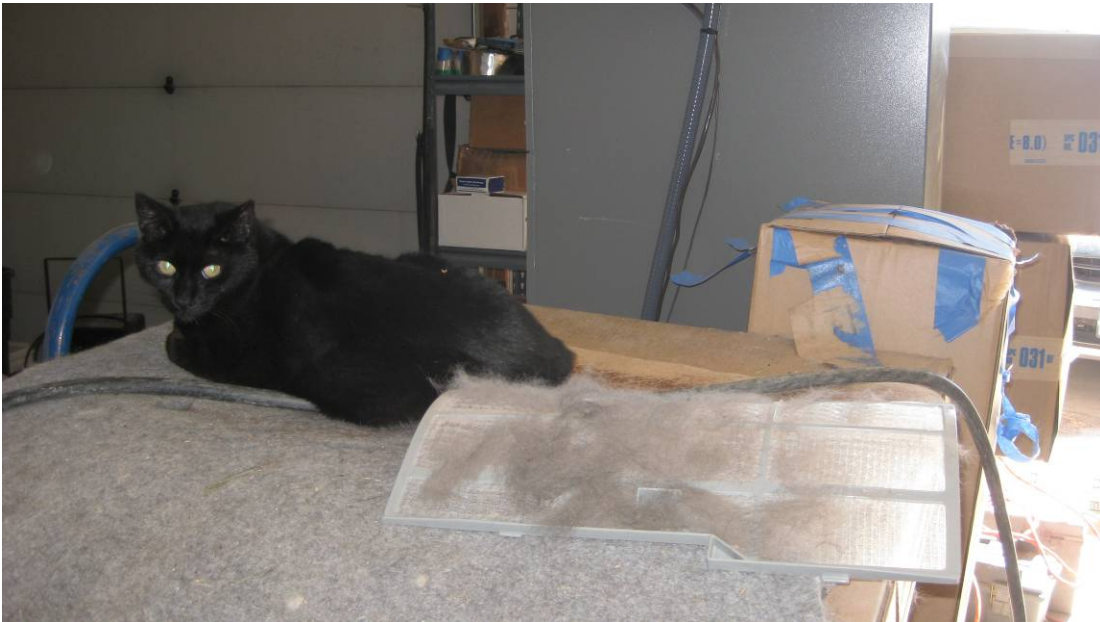
Figure 9. Partially Cleaned Filter and Source of Fouling
