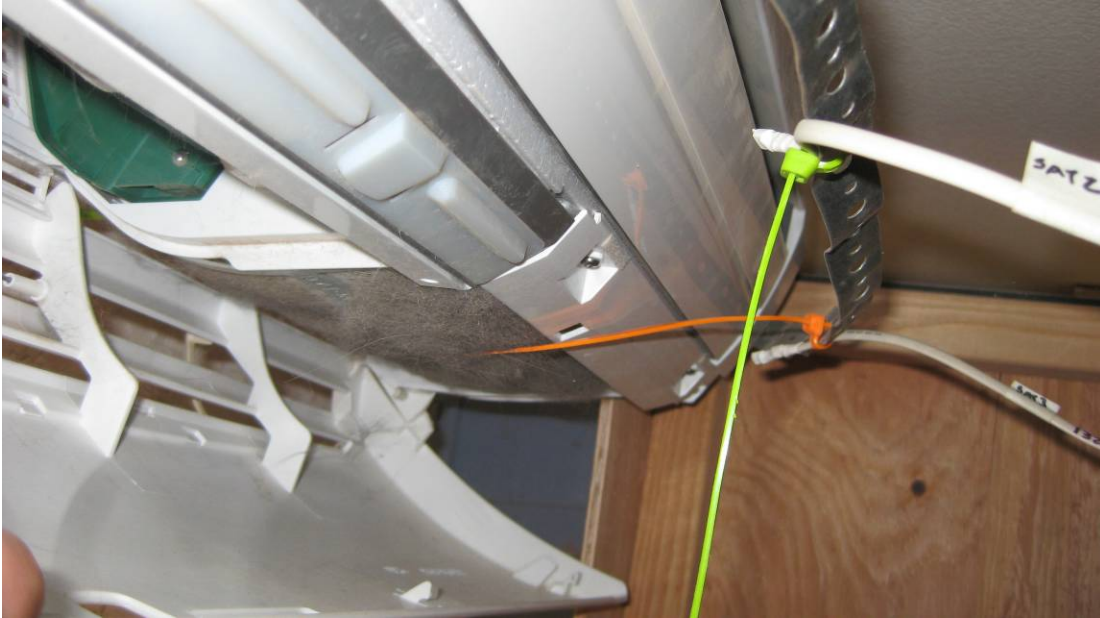
Figure 8. Fouled Filter in Place in Unit
