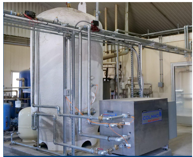
Commercial HPWH system with Colmac CxW-20.
