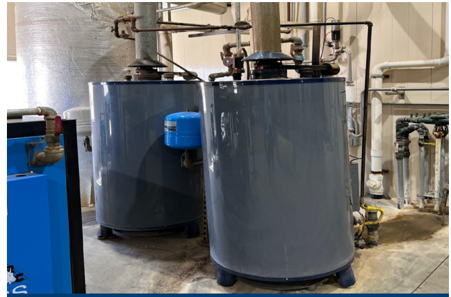
Original propane water heaters kept as backup.
