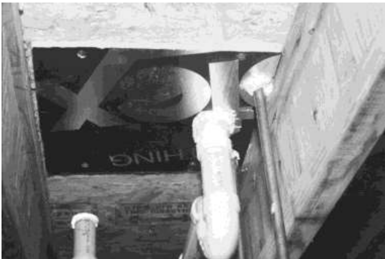
Sealing large plumbing penetrations: Foam board is attached with screws and washers. Gaps around the penetrations are filled with one-part foam to form a complete airtight seal.
