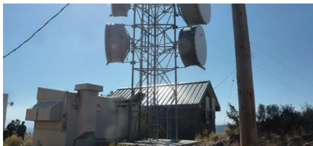
Tier X: Buck Butte Microwave Radio Station (1968) retains the original Armadillo Manufacturing Company control building; however, its function has been replaced by the new control building. The tower has also been replaced, and the site is not eligible for the National Register of Historic Places.
