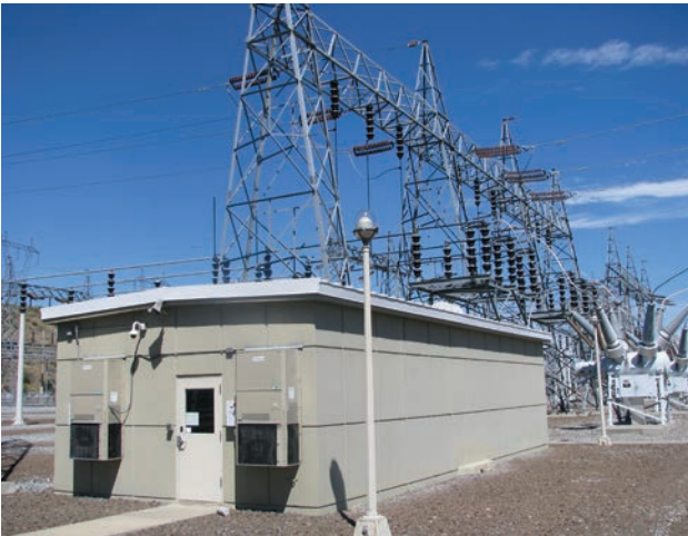
Relay house No. 1 at Chief Joseph Substation (1956) in Bridgeport, Washington.
