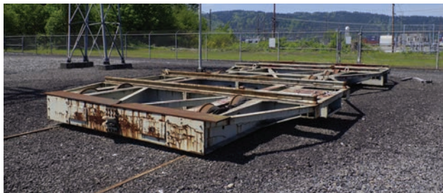
Transfer cart at St. Johns Substation.
