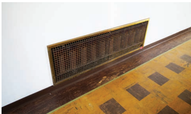
Brass radiator grill in St. Johns Substation Control House.
