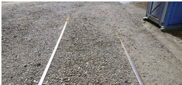
Transfer track at Salem Substation.
