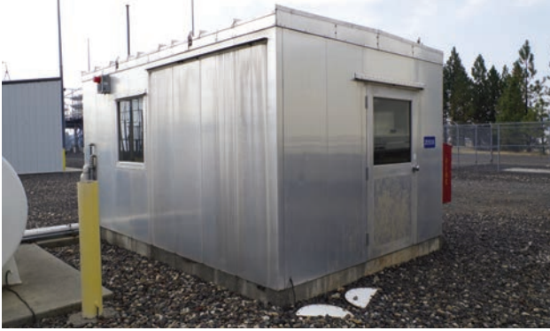
Engine generator building at Dworshak Substation.
