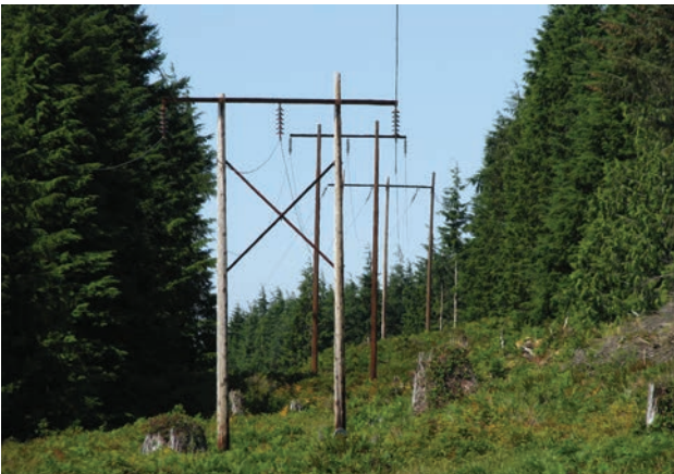
Holcomb-Naselle Transmission Line (1949) in southwestern Washington.
