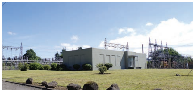
Tier II: Oregon City Substation (1941) in Oregon is historically significant in the areas of Commerce and Industry and supplied power to defense-related industries in Portland and the Willamette Valley during World War II.
