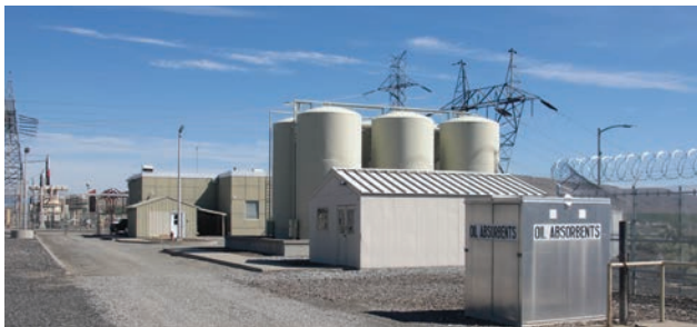
Tier II: Chief Joseph Substation (1956) in Bridgeport, Washington, is historically significant in the area of Government as representing the design, construction, operation, and expansion of BPA's transmission system during the System Expansion Period.
