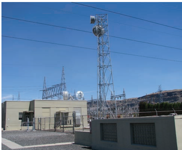
Columbia Substation (1945) in Rock Island, Washington, is significant in the area of Industry for supporting regional industrial development. The substation is also significant in the area of Commerce for delivering hydropower to Portland General Electric's commercial customers.
