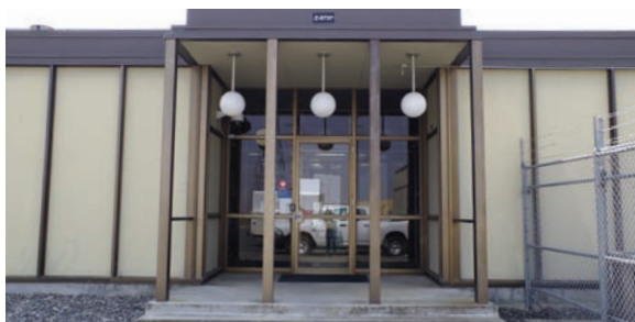
Modern Glass Globe light fixtures used at entrances during the 1960s.
