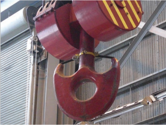
Untanking Tower crane for lifting and moving heavy equipment.
