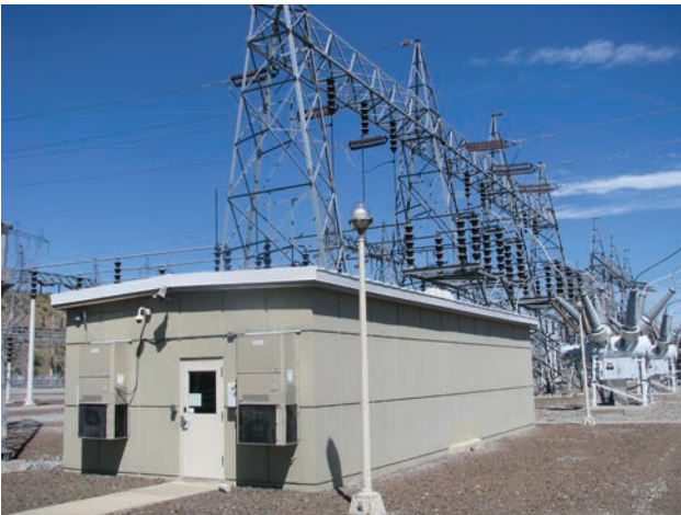
Chief Joseph Substation Relay House No. 1 (1956).
