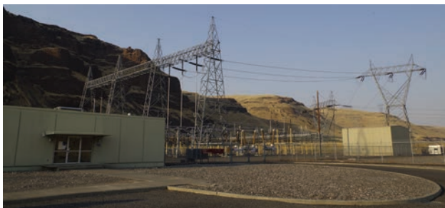
Little Goose Substation (1970) near Riparia, Washington, is significant in the area of Engineering for its association with the Pacific Northwest–Southwest Intertie.
