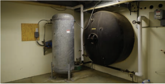
Hot water tank.
