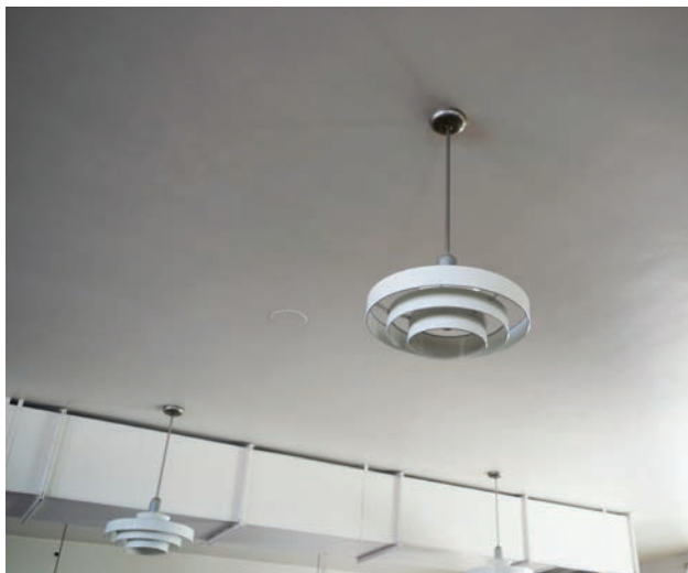
Streamline Moderne light fixtures at St. Johns Substation Control House.
