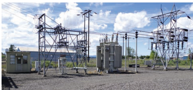
Tier III: Harrisburg Substation (1946), near Harrisburg, Oregon, is important for its association with rural electrification.
