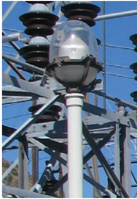
Switchyard light pole.
