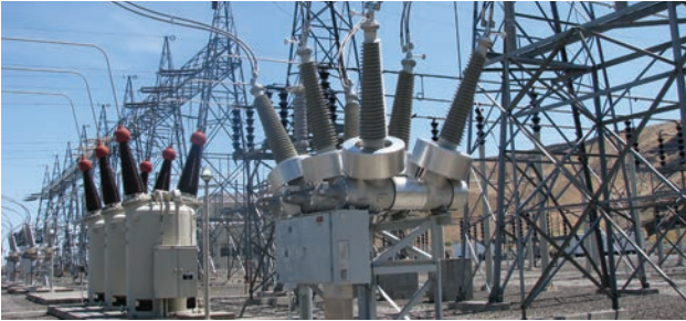
Switchyard with oil (left) and gas (right) circuit breakers at Midway Substation (1941).
