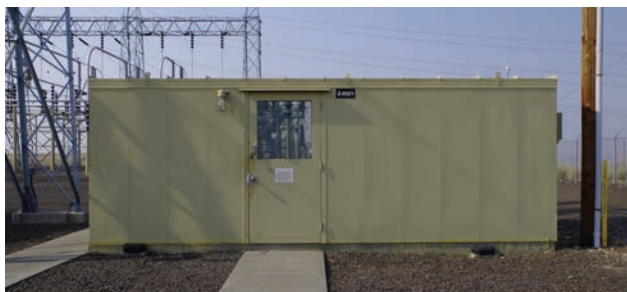
Utilitarian control house at Maupin Substation (1974) in Oregon.
