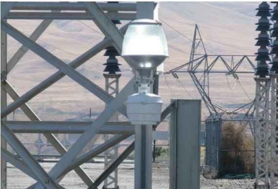
Switchyard light pole.
