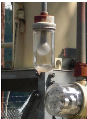
Switchyard light fixture.
