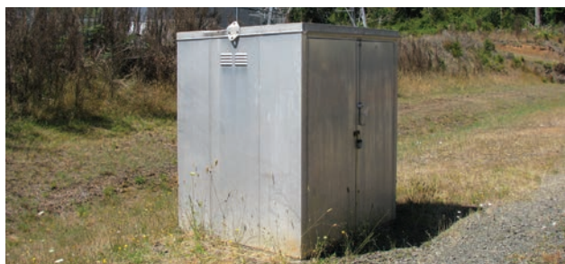
Pump house at Wendson Substation (1973) in Florence, Oregon.
