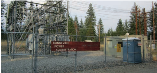
Tier II: Troy Substation (1953) in Troy, Montana, is historically significant in the areas of Commerce and Industry and represents BPA's expansion into western Montana during a period of tremendous growth.
