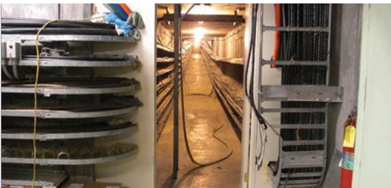
Cable tunnel housing underground cables between a control house basement and switchyard.
