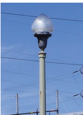
Switchyard light pole.
