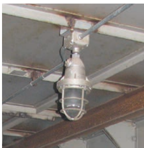
Utilitarian steel light fixtures. Murray Substation Control House (1972), left, and Midway Substation (1941), right
