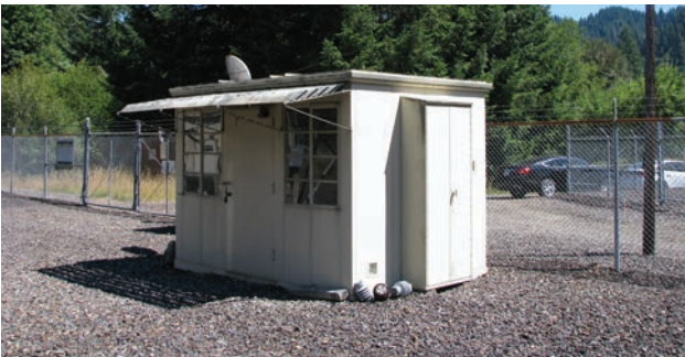
Walton Substation Control House (1949) is significant for reflecting BPA's use of standardized designs in substation development and for exemplifying BPA's Standard Aluminum Control House Type 190 model.
