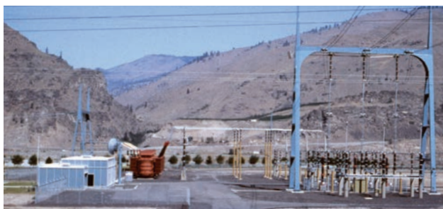
Sickler Substation, showing building and dead-end towers painted "BPA-1" Blue, 1970.
