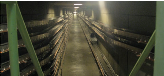
Cable tunnel access from control house basement at Boundary Substation (1967).
