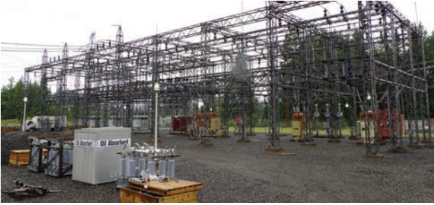
Switchyard at Chehalis Substation (1941).
