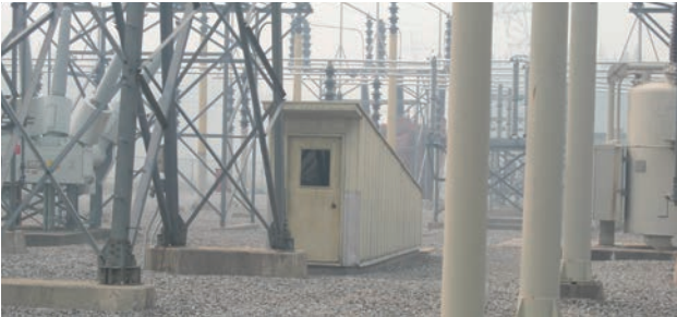
Cable tunnel access from switchyard at Boundary Substation (1967).
