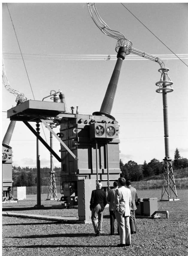
Figure 1. 230-kilovolt breaker at the Lyons Test Facility, September 8, 1977. 2
