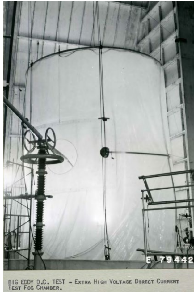
Figure 25. Interior fog test chamber within the Power Supply Building, ca. 1965. 149
