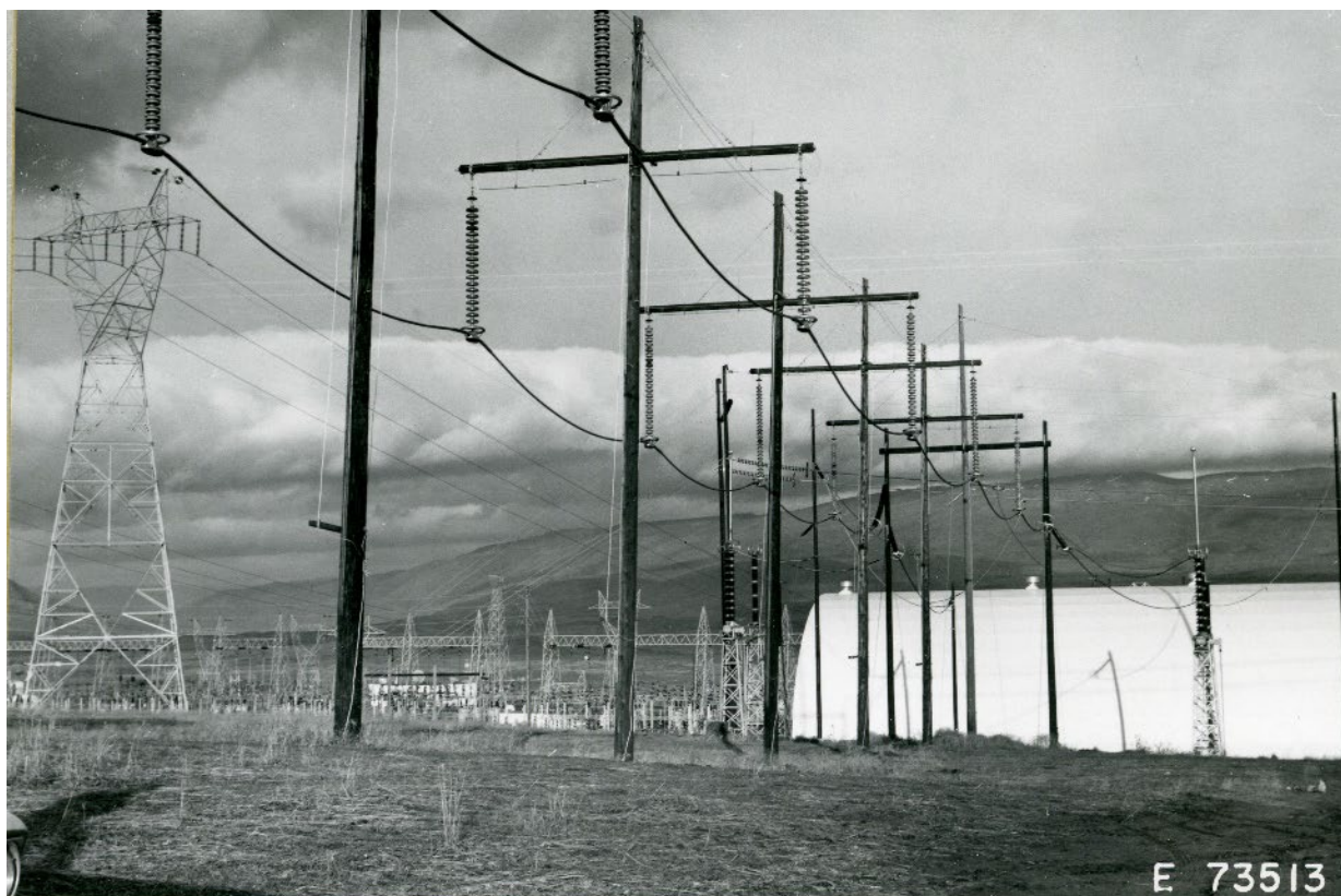
Figure 21. View of HVDC Test Center, including Insulator Leakage Line and Power Supply Building, 1964. 135
