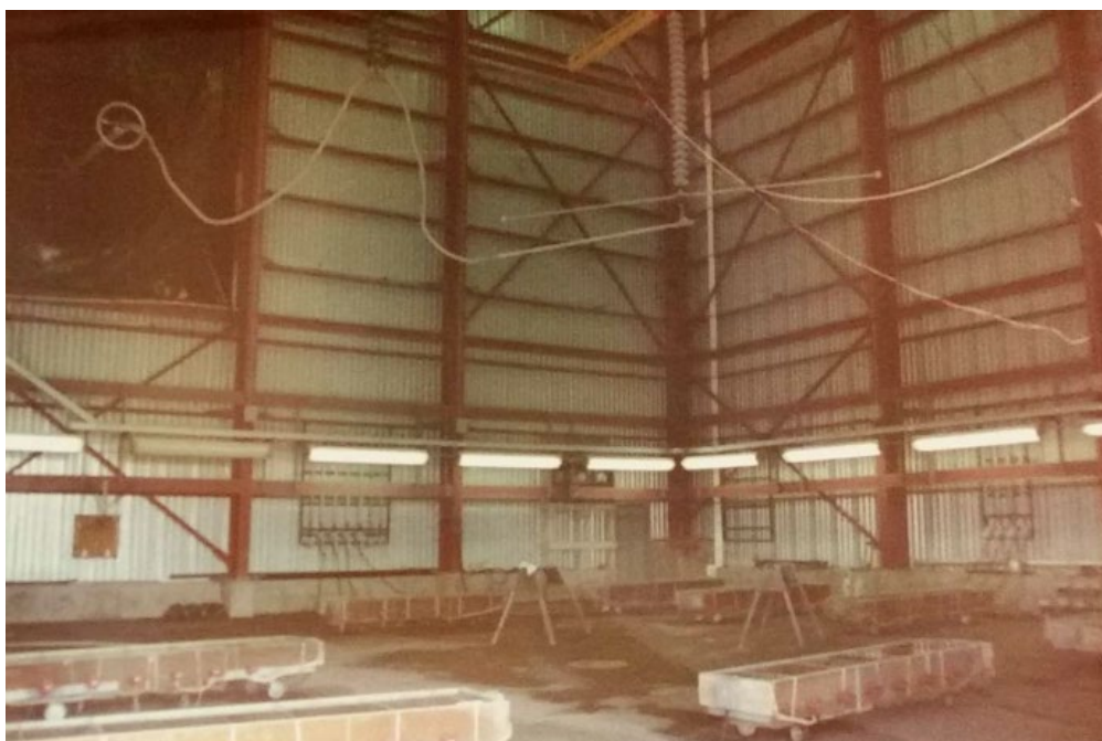
Figure 27. Interior of the Fog Chamber showing the metal tubs and hoists, ca. 1970s. 154
