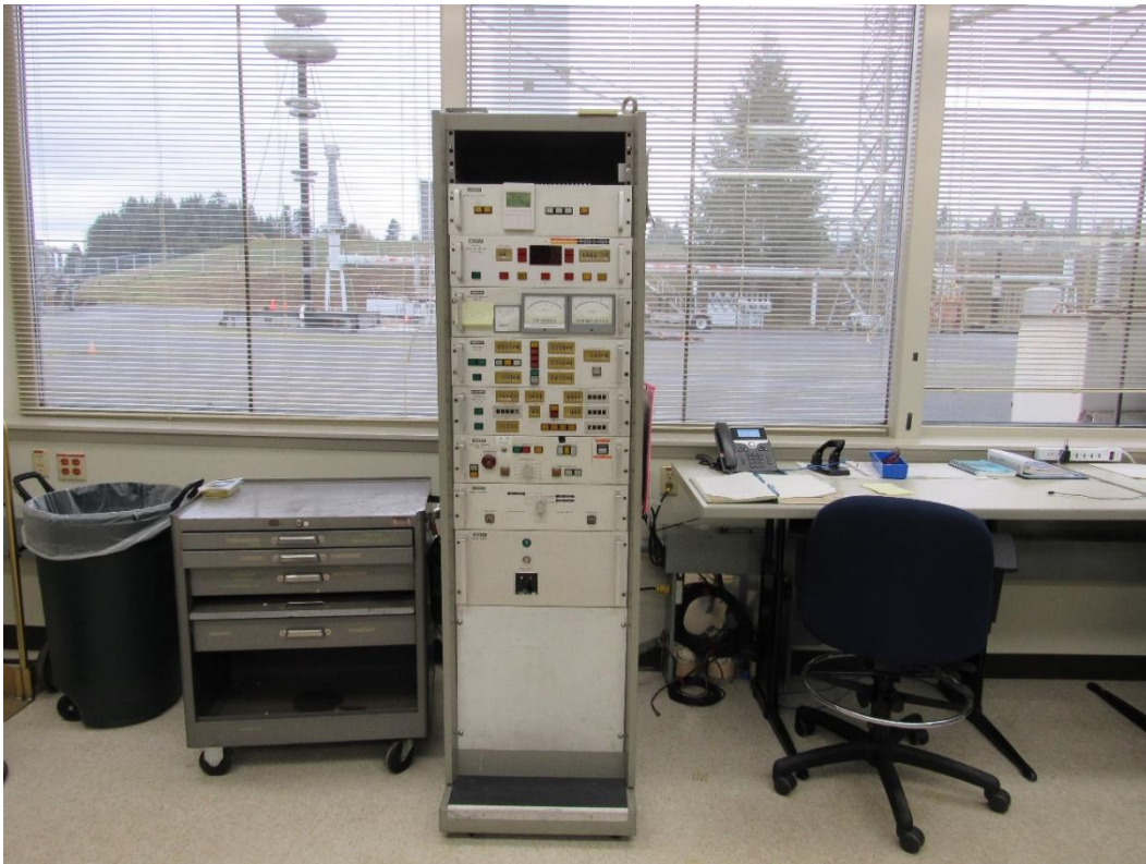
Figure 20. Photo inside the Motor Generator Lab looking out to the UHV Outdoor Test Yard. 131
