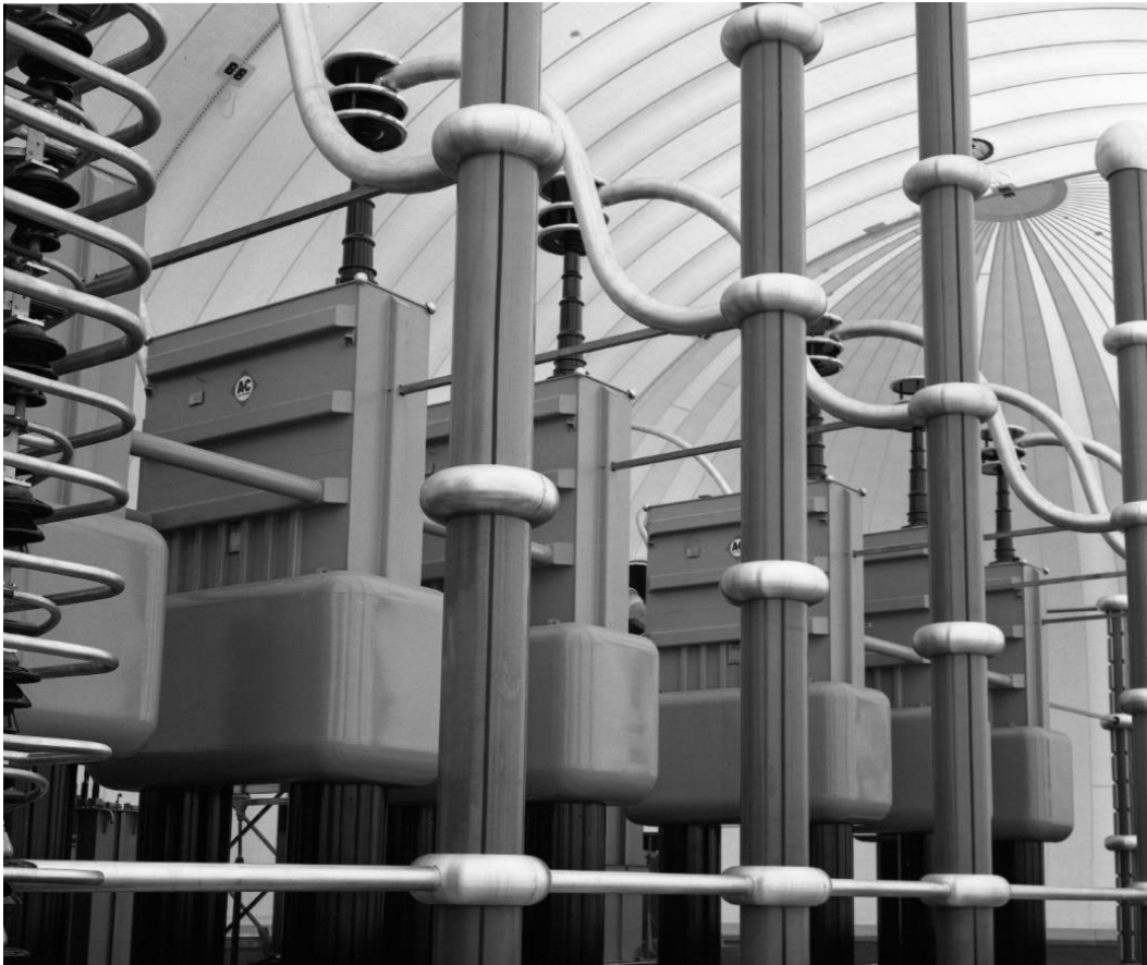
Figure 2. UHV testing equipment at Big Eddy HVDC Test Site, 1963. 39
