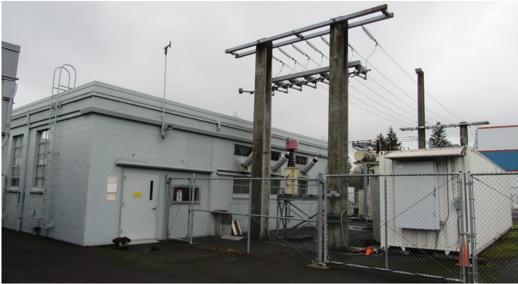
Figure 19. Medium Voltage Testing Building. 130
