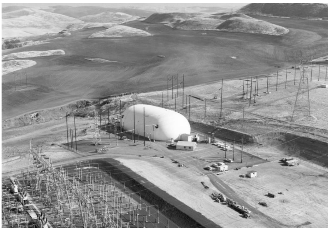
Figure 21. HVDC Test Center in The Dalles, Oregon, 1963. 141
