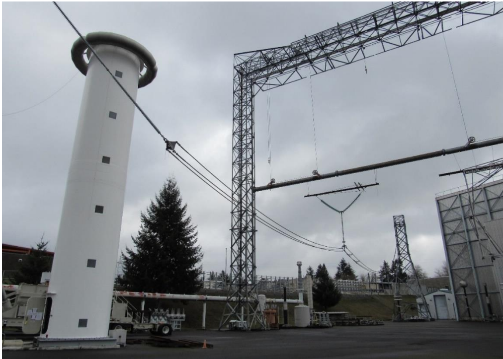
Figure 10. Impulse Generator (left) in the UHV Outdoor Test Yard. The Portal Test Tower is visible to the right. 109
