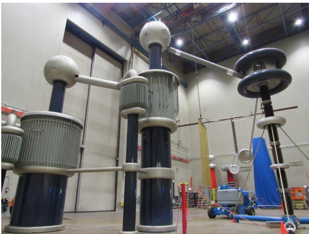
Figure 6. The cascade transformer and large 60-foot utilitarian doors (background). 91
