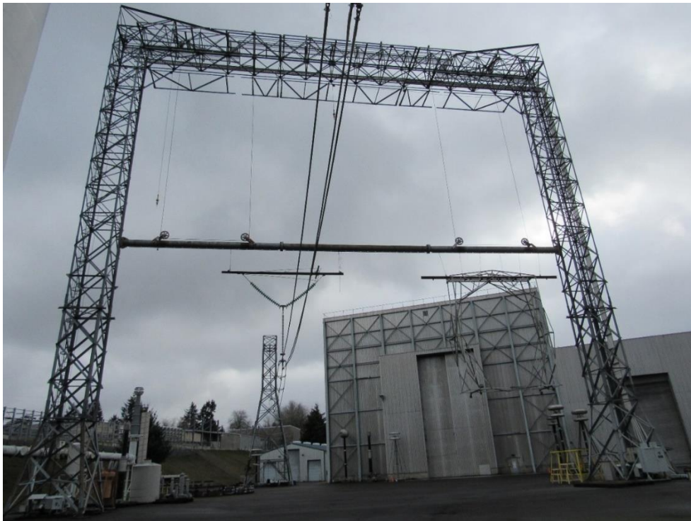
Figure 12. Portal test tower with Carey UHV Lab visible in the background. 111
