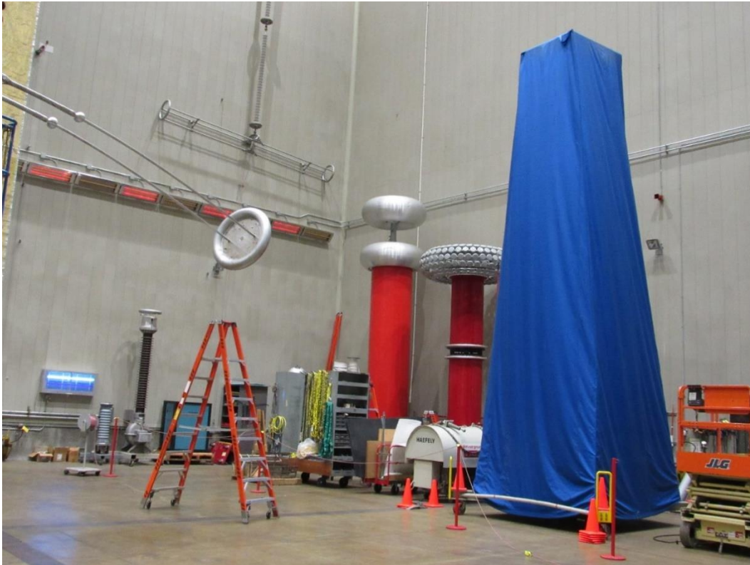
Figure 7. Impulse generator (underneath blue tarp) and DC voltage divider and capacitor (two red towers to the left of the impulse generator). 96
