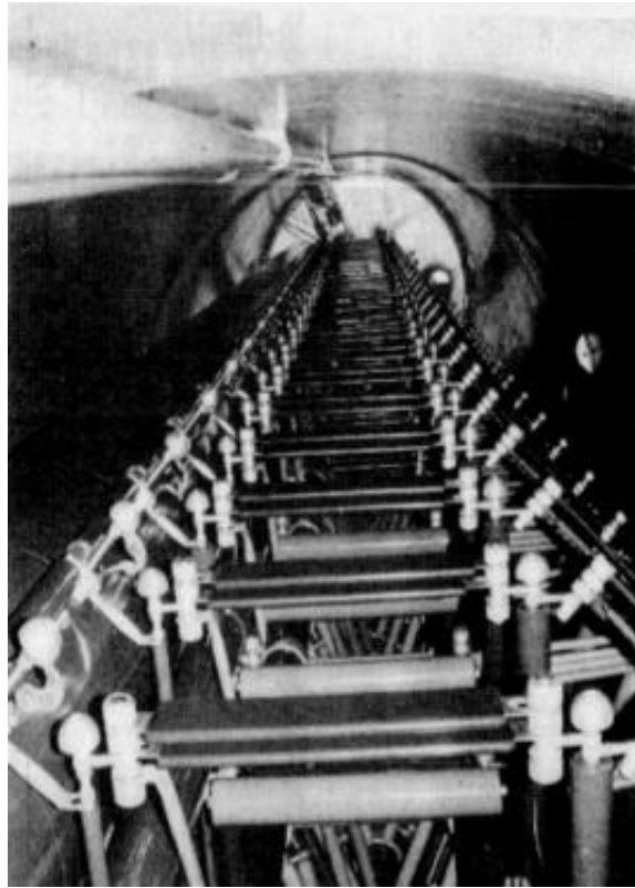
Figure 11. Interior of the outdoor pulse generator. 110
