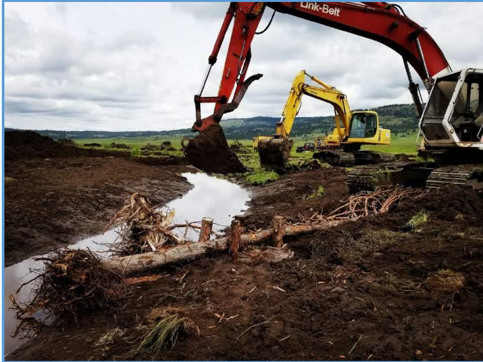
2018001 Fox Creek Structure Placement resulted in turbidity
