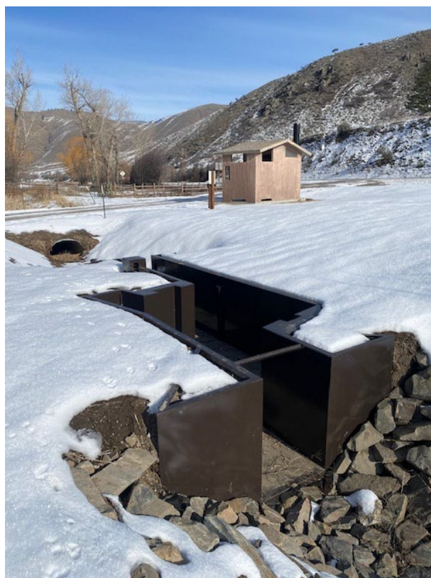
Figure 40. 2025012: IDFG steel modular fish screen.
