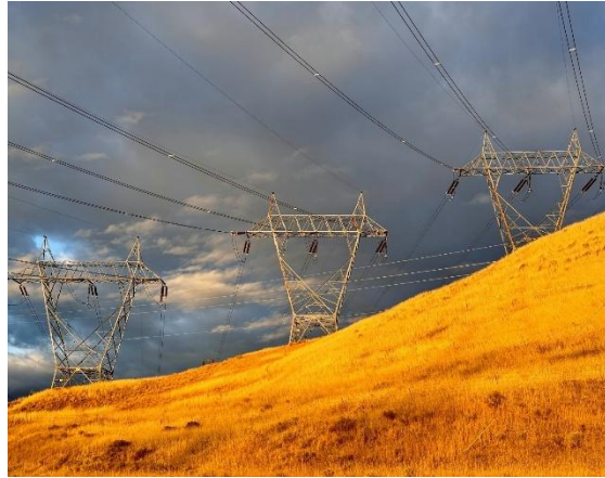
BPA transmission structures near Rufus, Oregon. (Photo by Rob M.)
