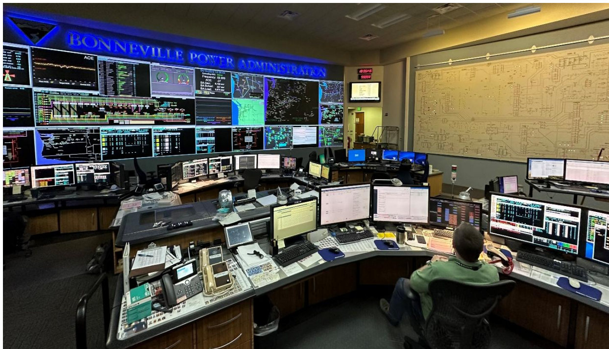
BPA control center.
