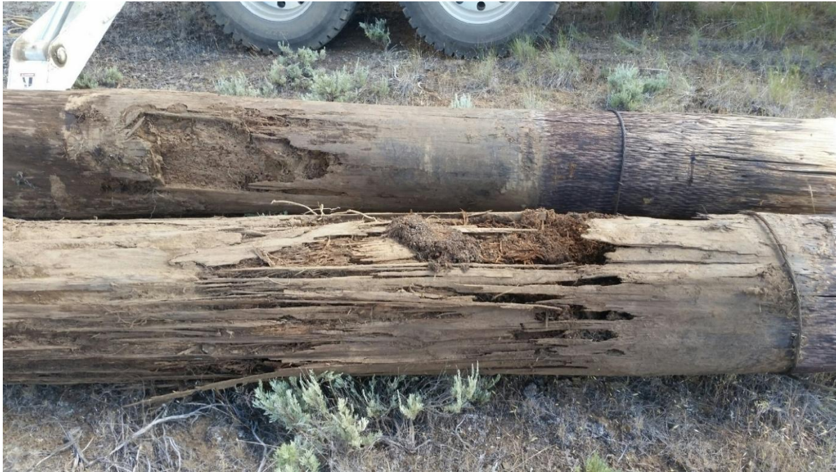
Wood pole decay.
