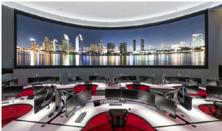
CONFIDENTIAL CALIFORNIA POWER UTILITY - GRID CONTROL
