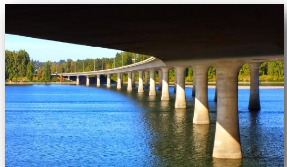
Underside view of the I-205 Glen Jackson Bridge, which crosses the Columbia River
