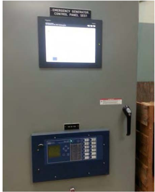
Existing Emergency Diesel Generator Control
