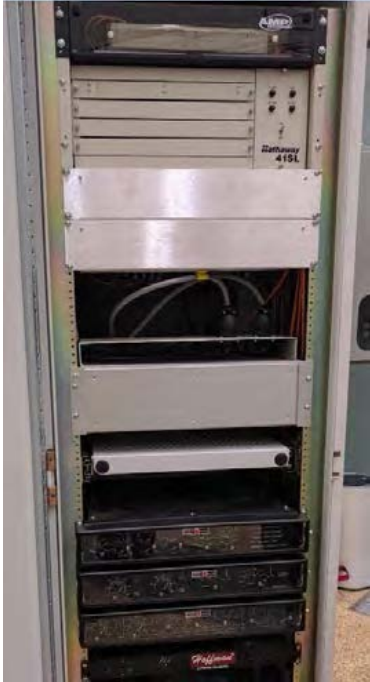
Existing Synchronizer and Hathaway SER system
